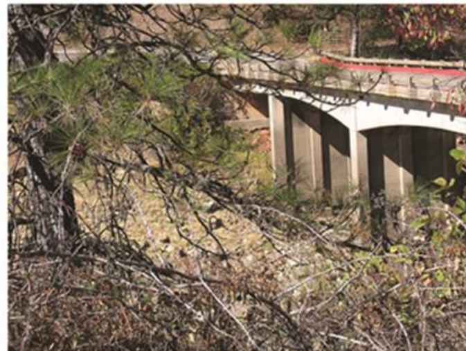
McCloud Arm VAU, KOP 16, Photo 16 View of the McCloud River Bridge, from the eastern approach.
