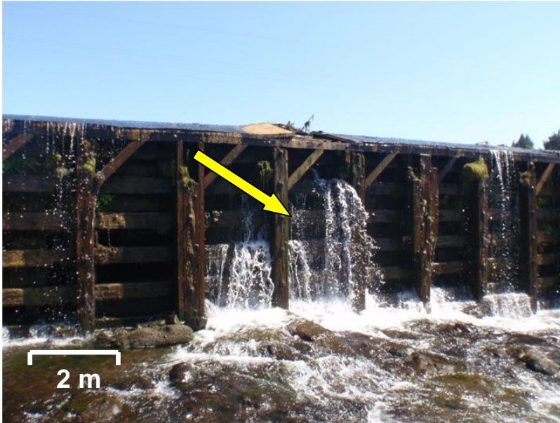
Figure 3.9. The enlarged opening on the surface of Winchester Dam during the first day of the reservoir dewatering event on 31 August, 2009. Within an hour after this photo was taken, many adult Pacific lamprey began to retreat from within the timber crib structure (arrow symbol), totaling over 250 adults this day.
