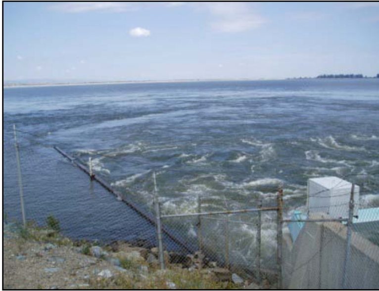
Figure 54. Clifton Court Forebay showing turbulence behind the radial gates. Photo by Dave Vogel.
