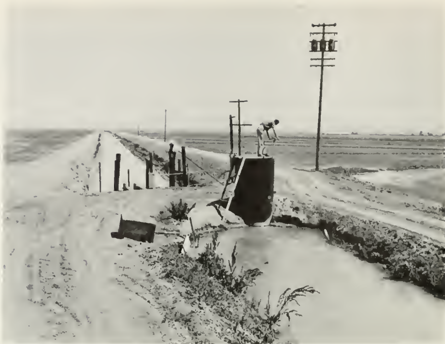
Many of the pumps are located on feeder canals some distance from the main drainage canal.
