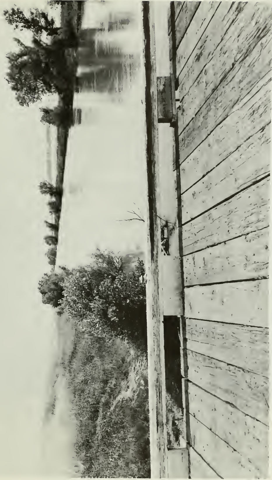
Colusa Basin Drainage Canal showing back levee of R. D. 108 on left (east). No levee protection on right (west).
