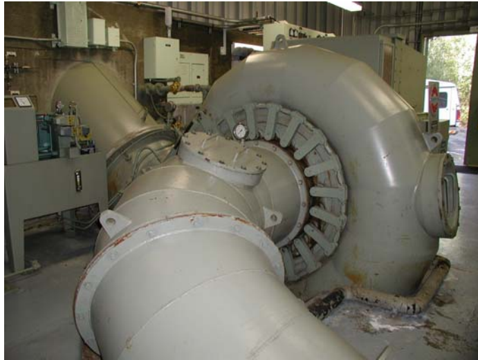
Volta 2 Powerhouse—Hydroelectric Turbine
