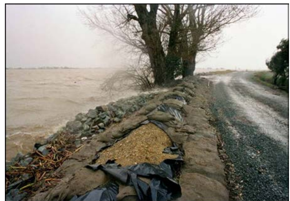
Levee damage during a storm
