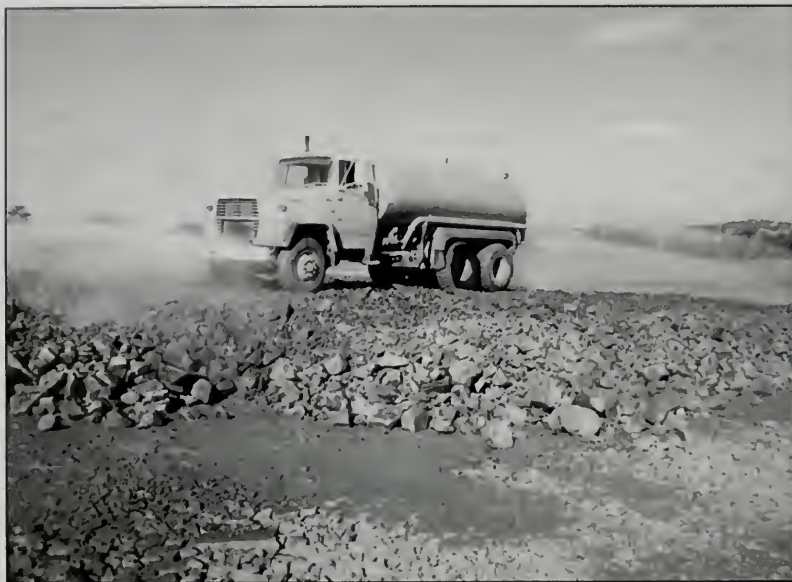
Figure 2. Significant moisture being added during fill placement.
