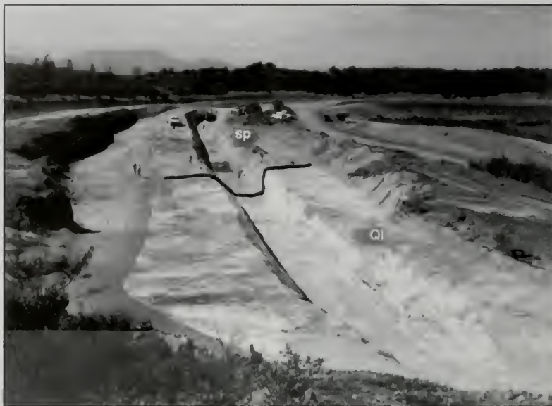
Figure 5. The excavation for the enlargement of the Homestake Tailings Dam encountered an unexpected occurrence of Quaternary lake deposits (Ql). Since the foundation objective called for highly weathered serpentinite (sp) rock, the unconsolidated silty deposits required visual examination to determine their adequacy. The fault contact between the serpentinite and the lake deposits was demonstrated to be inactive before fill placement could begin. [File photo by the author.]
