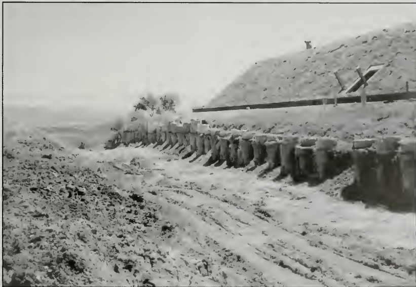
Figure 10. A portion of a tied-back, reinforced concrete shear pin wall installed at the Codorniu Napa site to protect the upslope winery facilities. This shear pin wall roughly follows the alignment of cross-section 1 shown in Figure 7.
