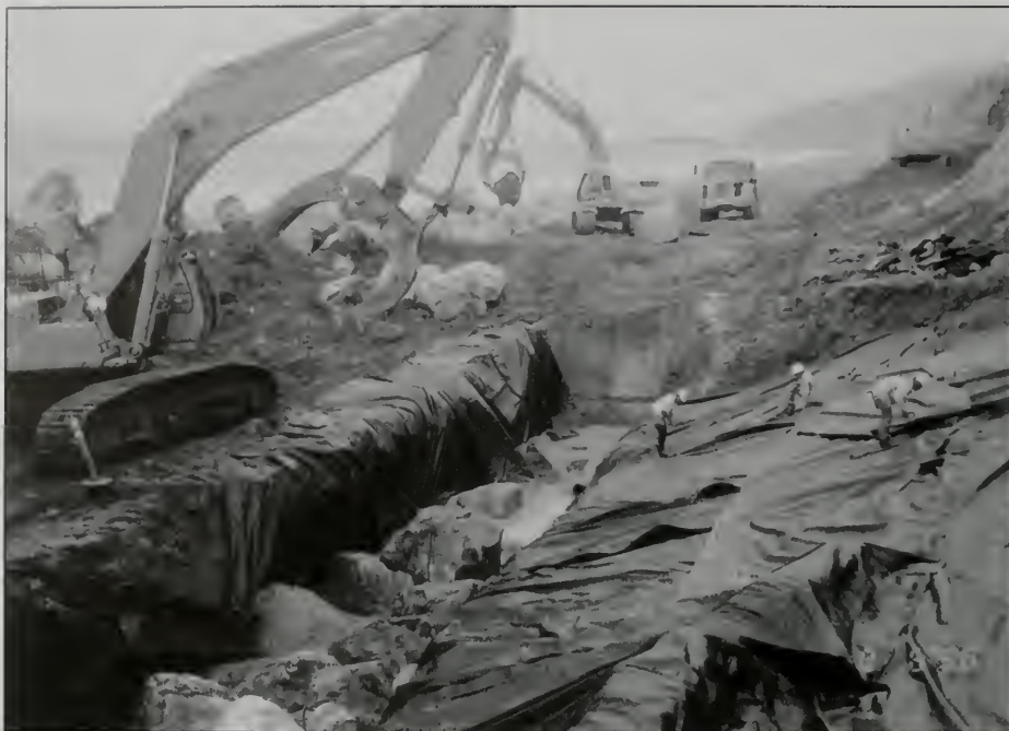
Figure 8. Filter fabric is being placed in the keyway and along the base of the revetment prior to stone placement.
