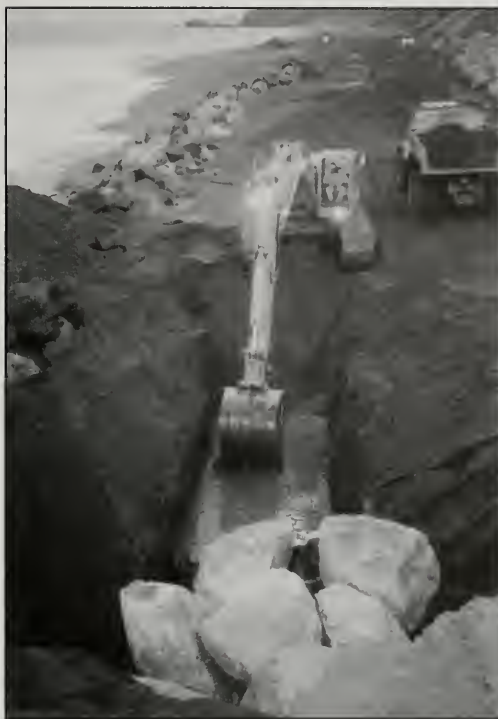
Figure 9. Keyway excavation below mean sea level required strategic construction timing with respect to tidal conditions.
