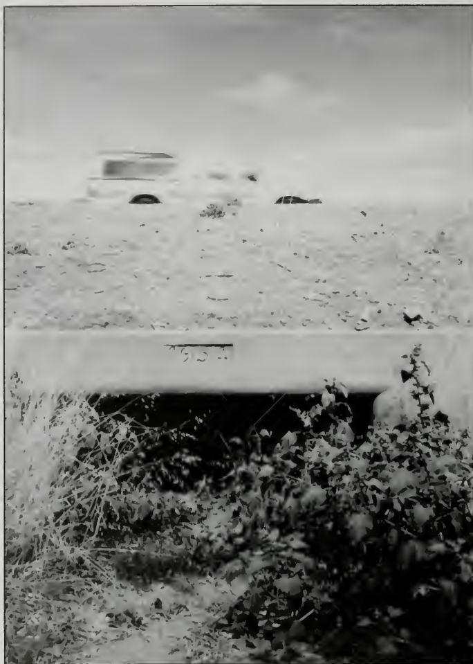
Figure 8. The upstream (northeast) side of the 1954 Freeway culvert almost completely plugged with Orchard Creek sediments.
