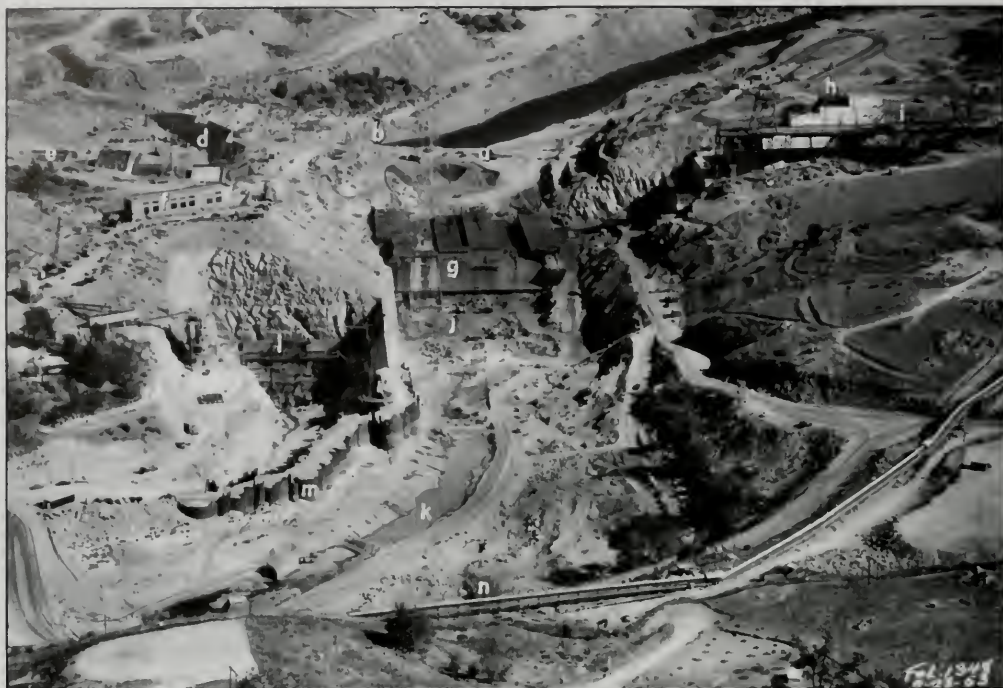
Figure 7. Aerial oblique view of the concrete gravity dam. Folsom Project under construction, showing the principal engineering features and related activities (9/28/53): (a) upstream cofferdam; (b) intake, diversion tunnel; (c) spoil area; (d) retaining wall to hold back earth-fill wing dam; (e) wing or abutment blocks (monoliths); (f) pumping plant; (g) river section of gravity dam, note monoliths (overpour spillway design); (h) wing or abutment monoliths; (i) trestle used to place concrete; (j) stilling basin; (k) tailrace; (l) power house in deep excavation, showing partial underground design; (m) sheet-piling; (n) conveyor belt, transporting concrete aggregate from pit to batching plant (from Kiersch, 1955).
