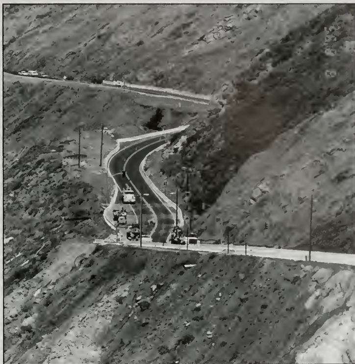
Figure 13. View of the reconstructed section, which was completed on June 30, 1995. Photograph by Robert Colin.
