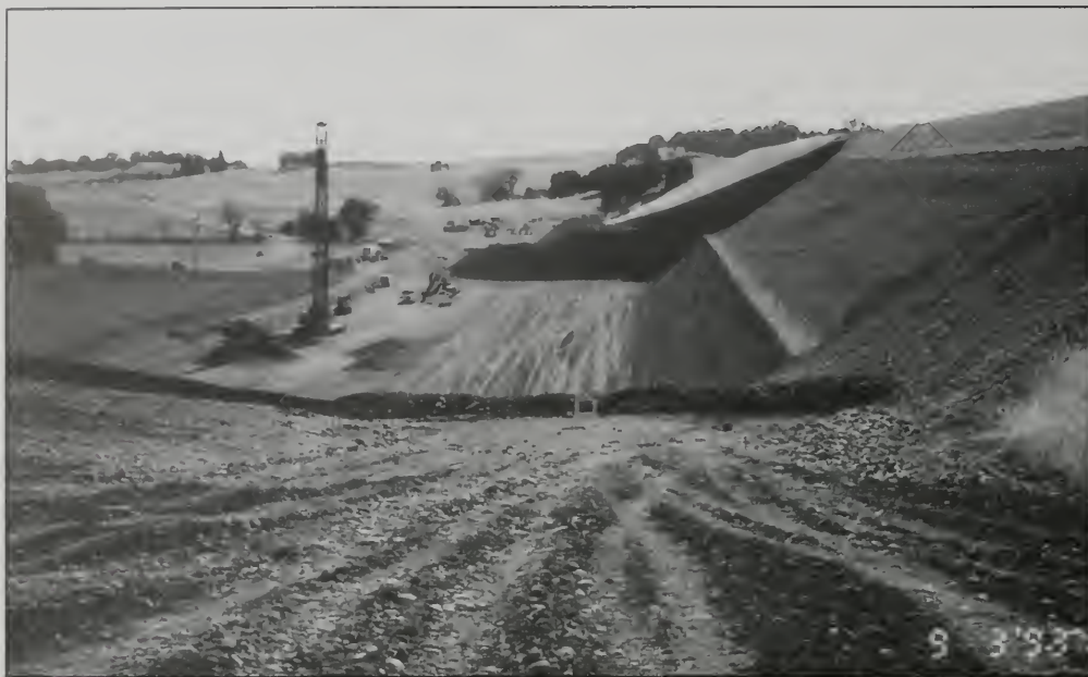
Figure 6. Downstream seismic remediation of the Mormon Island auxiliary dam – Embankment excavation and working surface for bottom-feed stone columns and mini-columns.
