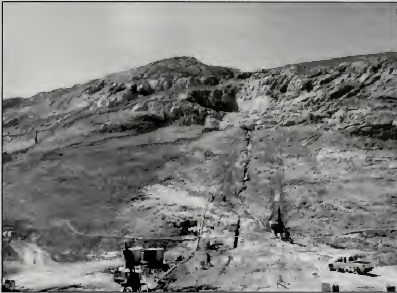
Figure 2. Channel section and left abutment of Los Vaqueros Dam. The foundation objective of moderately weathered or better rock of the Panoche Formation has been reached in the channel section, the cutoff wall is completed, and curtain grouting is underway. Additional excavation was needed on the left abutment to obtain an acceptable foundation. [File photo by the author.]
