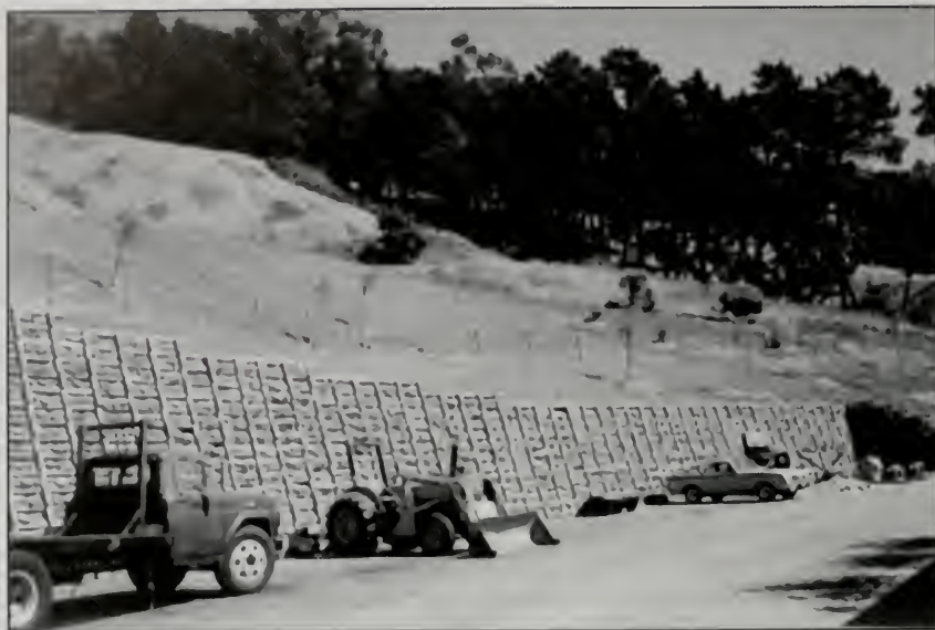
Figure 5. Parking lot slope retention. This photograph, taken at the completion of the project, shows the earth buttress fill above a crib wall. View is to the southeast. The main trace of the Hayward fault crosses the parking lot at the extreme lower right hand corner of the photograph.
