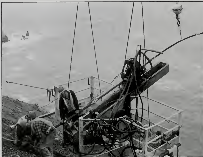
Figure 12. Seventy rock anchors, up to 60 feet in unbounded length, were installed at three levels below the roadway. Photograph by Robert Colin.
