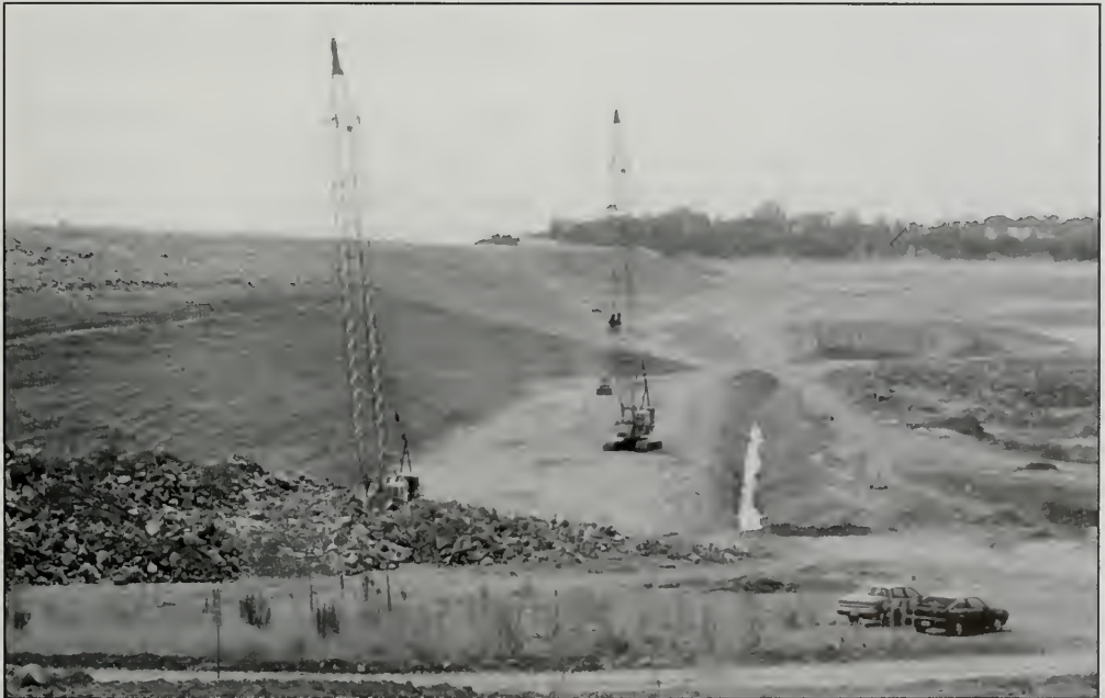
Figure 4. Upstream seismic remediation of the Mormon Island auxiliary dam – Embankment excavation and working surface for dynamic compaction.
