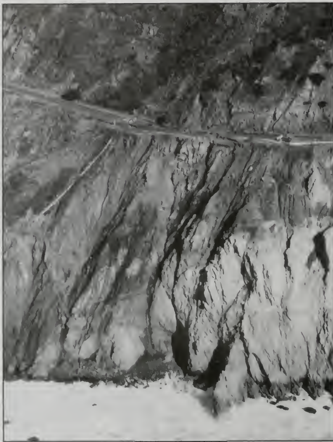
Figure 9. Offshore view of the slide. The dropped block was not only severely broken, but was also undermined in several areas, with the roadway unsupported. Photograph by Robert Colin.
