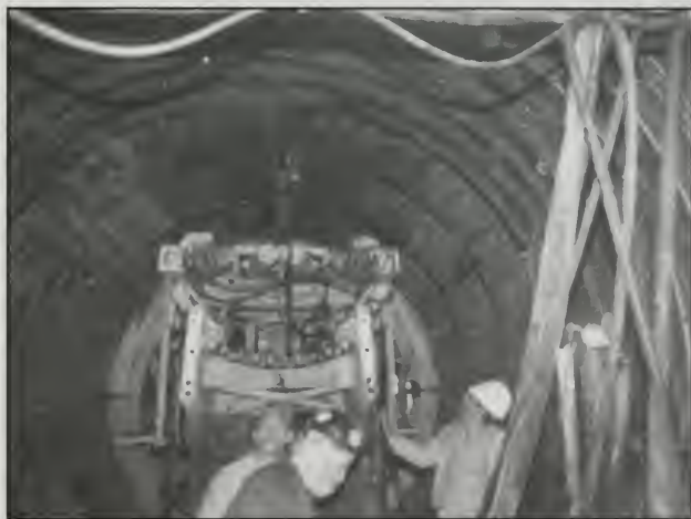
Figure 19. Initial tunnel lining. Steel ribs and wood lagging tunnel support are clearly shown.
