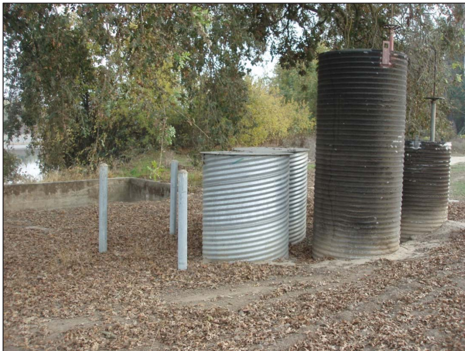
Figure 4: Maxwell Irrigation District, Corrugated ventilation tubes, view looking southeast (C. Jimenez, November 13, 2012).
