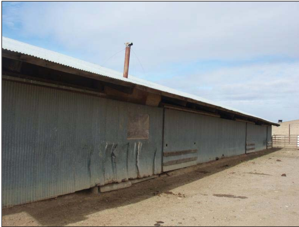
Figure 31: Edward Owens Farmstead, Lambing barn, east elevation, view looking northwest (C. Jimenez, November 13, 2012).
