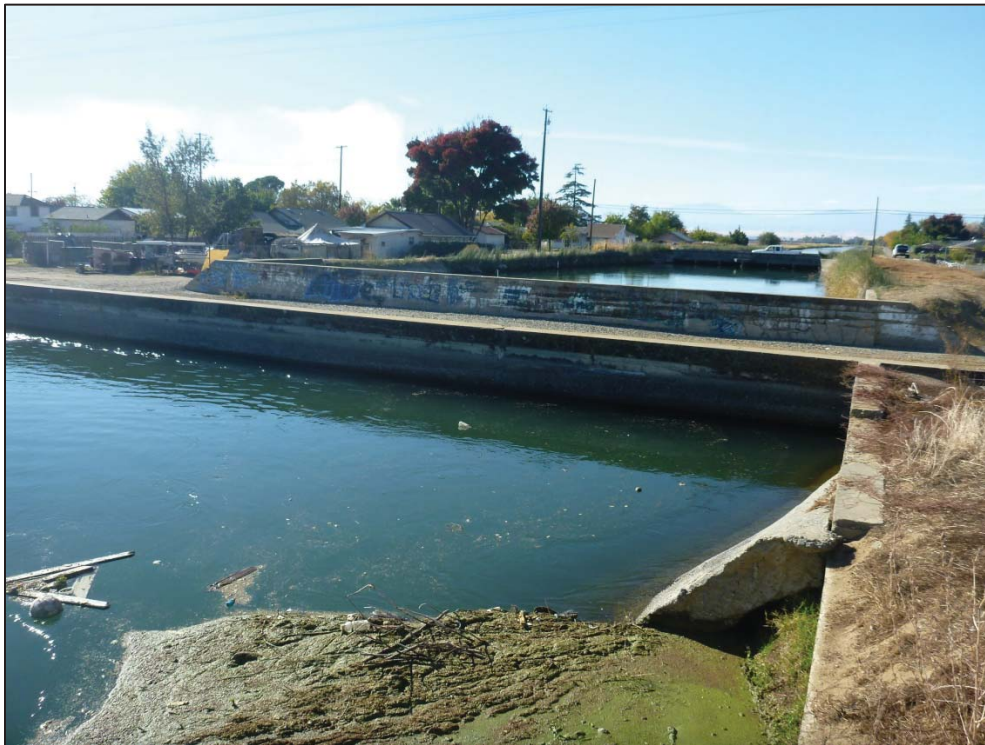
Figure 3: Union Pacific Railroad siphon looking at Highway 99W bridge, view looking southwest (C. Jimenez, November 14, 2012).
