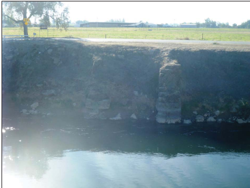
Figure 12: GCID remains of historic headgate, view looking west (C. Jimenez, November 14, 2012).
