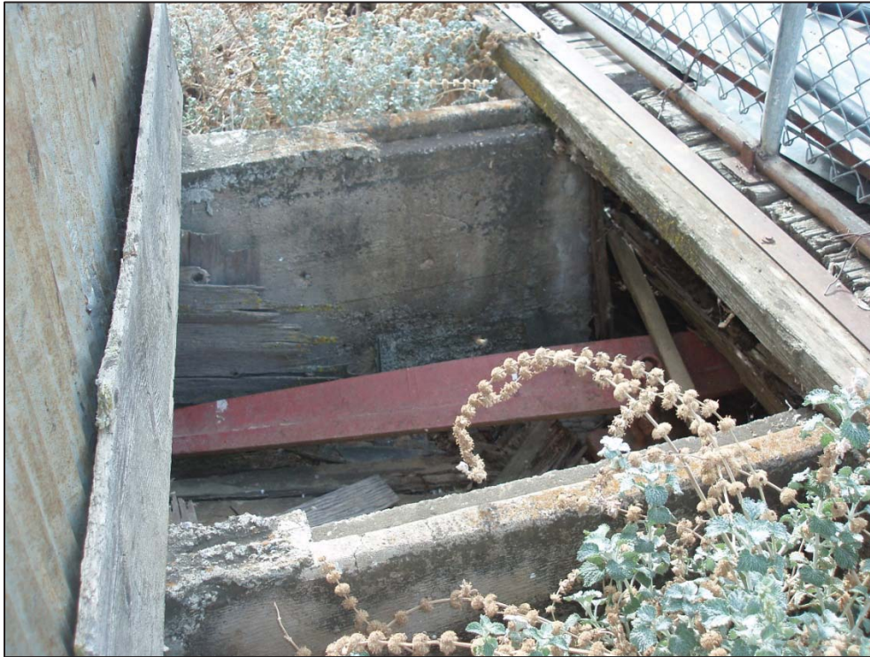
Figure 11: Shirley Jensen Farmstead, connector between shop and scale, view looking south (C. Jimenez, November 13, 2012).
