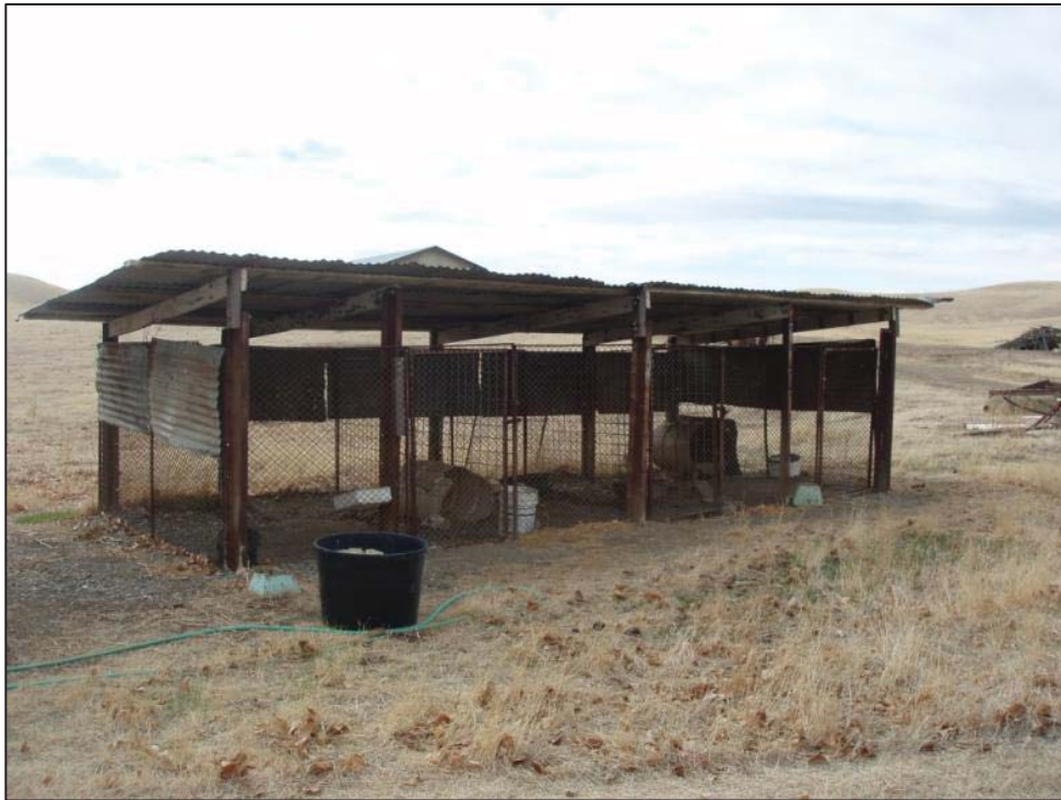
Figure 23: Edward Owens Farmstead, Western dog kennels, view looking west (C. Jimenez, November 13, 2012).
