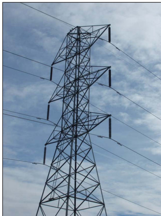
Figure 4: WAPA Maxwell-Olinda 500kV Transmission line, example of eastern tower (C. Jimenez, November 13, 2012).
