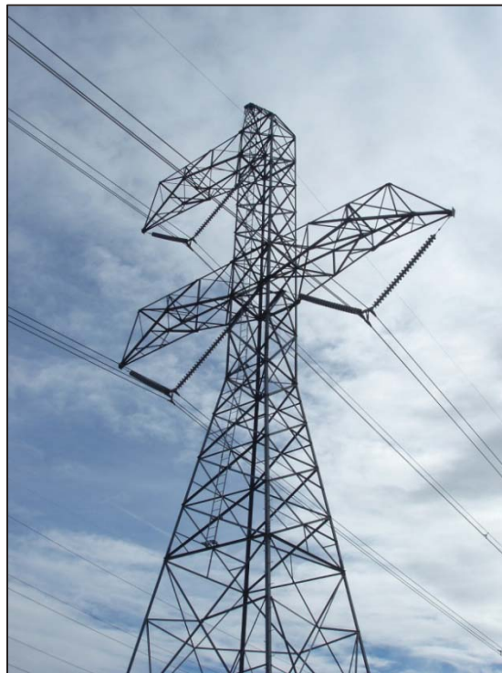
Figure 3: WAPA Maxwell-Olinda 500kV Transmission line, example of western tower (C. Jimenez, November 13, 2012).
