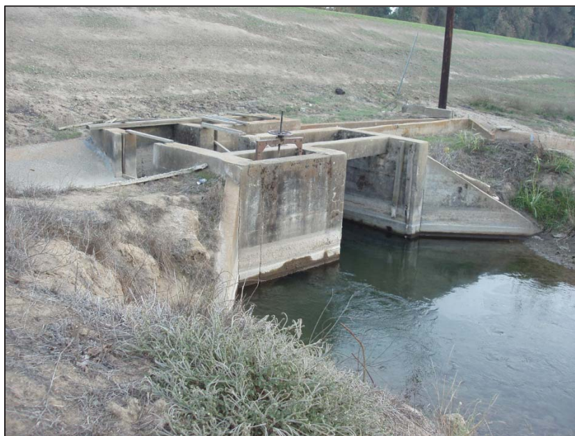
Figure 8: Maxwell Irrigation District, Concrete irrigation valve near the levee, view looking southeast (C. Jimenez, November 13, 2012).
