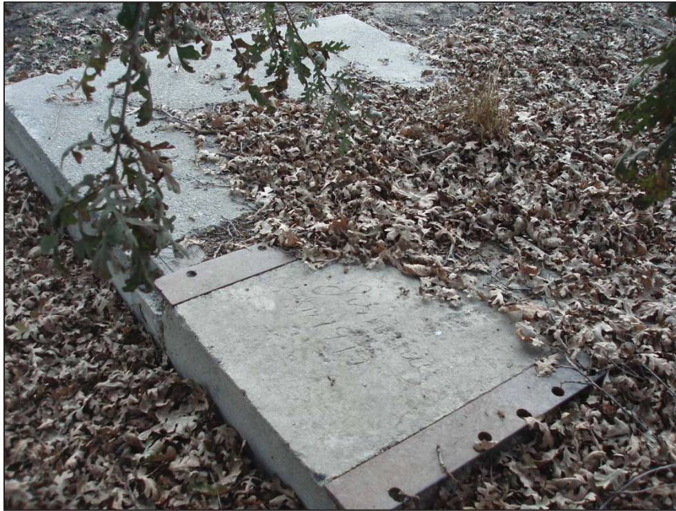
Figure 5: Maxwell Irrigation District, Concrete lid, detail (C. Jimenez, November 13, 2012).
