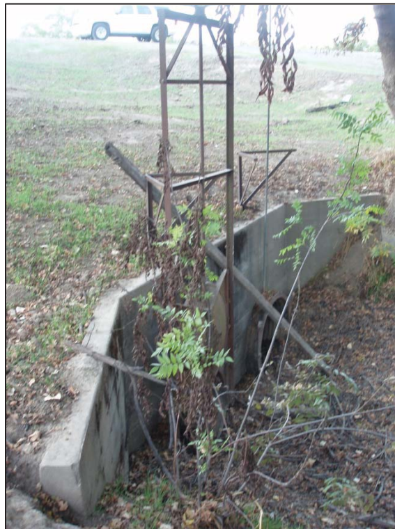
Figure 15: Maxwell Irrigation District, Concrete valve and culvert, view looking southeast (C. Jimenez, November 13, 2012).
