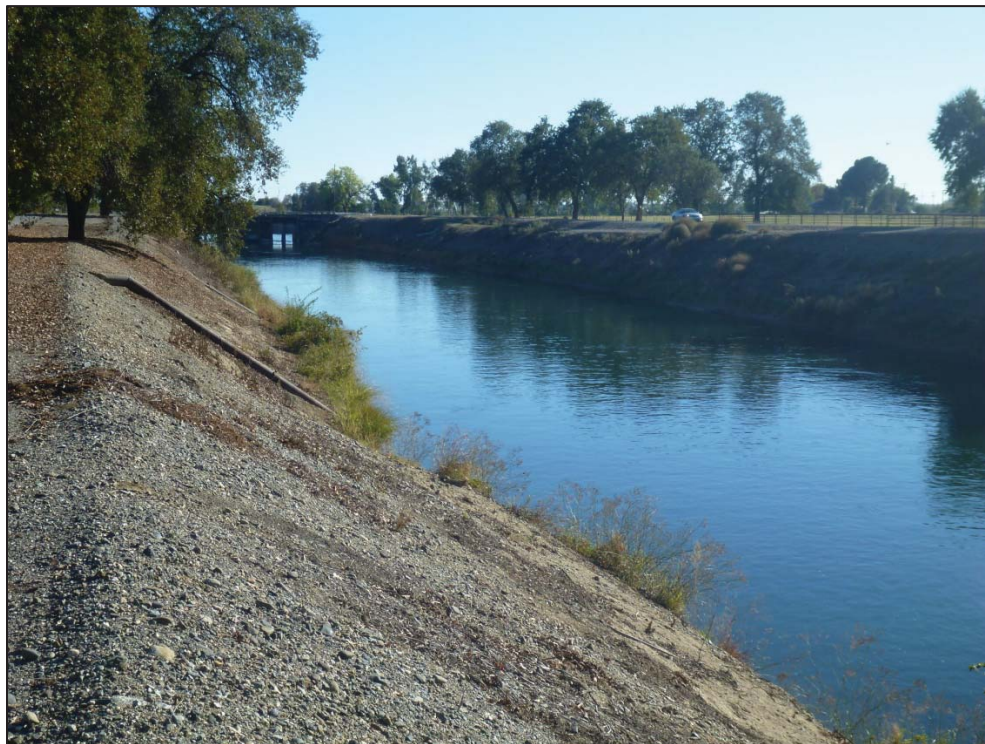
Figure 7: GCID Canal prism, view looking southwest at Headgate (C. Jimenez, November 14, 2012).
