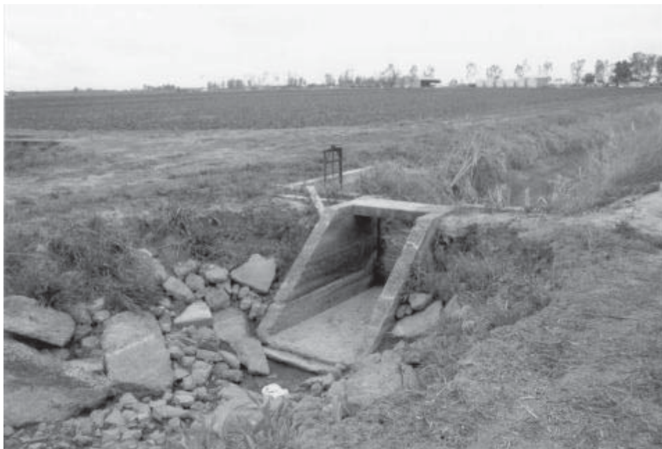
Photo 3. View of typical ditch and concrete diversion structure located on east side of McDermott Road south of Delevan Road; 6 March 2001. DB 1:5. Denise Bradley, photographer.
