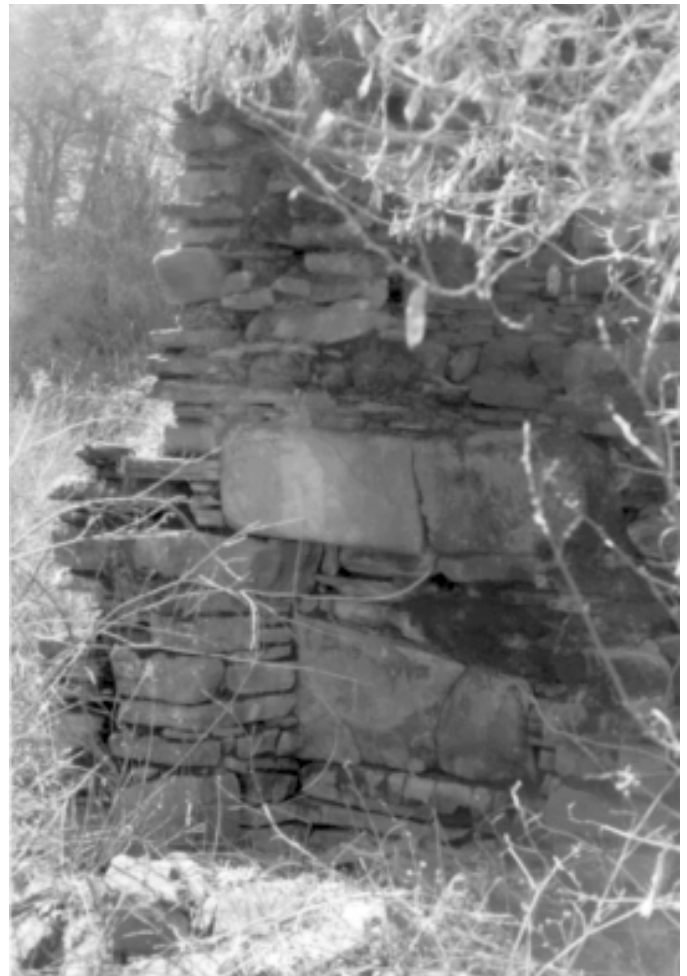
Figure 44: Sandstone Chimney at site SR-007-C.
