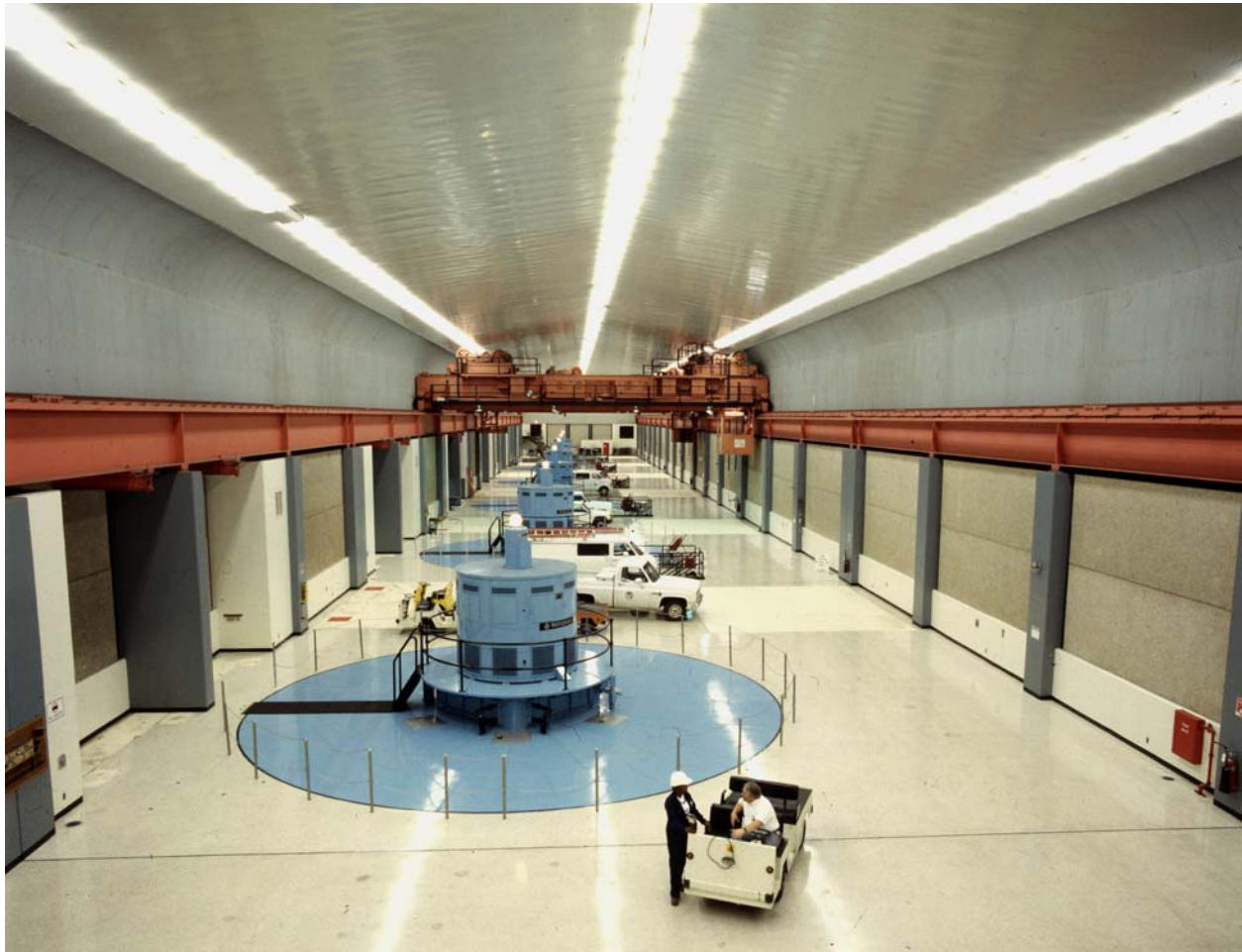
Figure A.2.1-2. Hyatt Pumping-Generating Plant.
