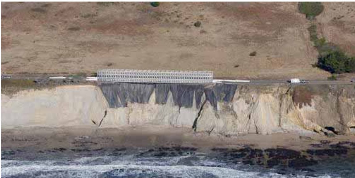
Figure 36. Road erosion along Highway 1 with deployment of erosion mitigation strategy
