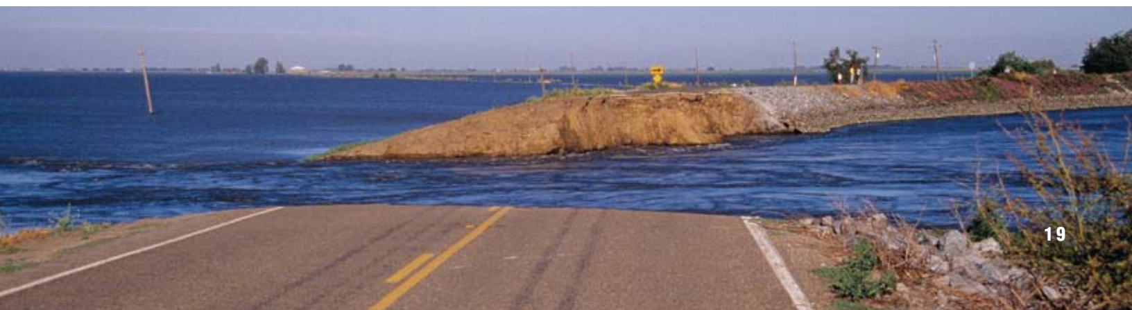
Levee break at Jones Tract
