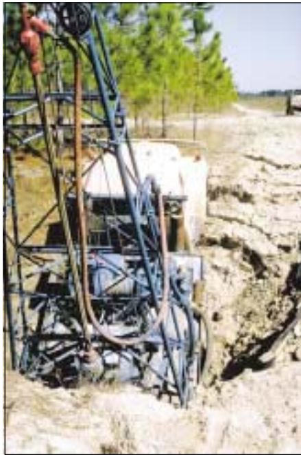
Figure 22. "A giant sink hole opened up on Thursday, September 19 [1975] at a drilling site near Tampa, Florida and swallowed up a well-drilling rig, a water truck, and a trailer loaded with pipe all valued at $100,000. The well being drilled was down 200 ft when the ground began to give way to what turned out to be a limestone cavern. Within 10 minutes all the equipment was buried way out of sight in a crater measuring 300 ft deep, and 300 ft wide. Fortunately, the drilling crew had time to scramble to safety and no one was hurt." -from National Water Well Association newsletter. (Photograph courtesy Tom Scott.)
