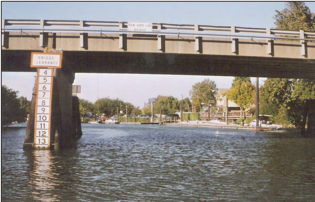
Figure 5.5-3. View of New Hope Bridge from the South Fork of the Mokelumne River, looking north. Note Wimpys/New Hope Marina complex visible beyond bridge. This bridge would be subject to retrofit or replacement under Alternatives 2-A through 2-C.
