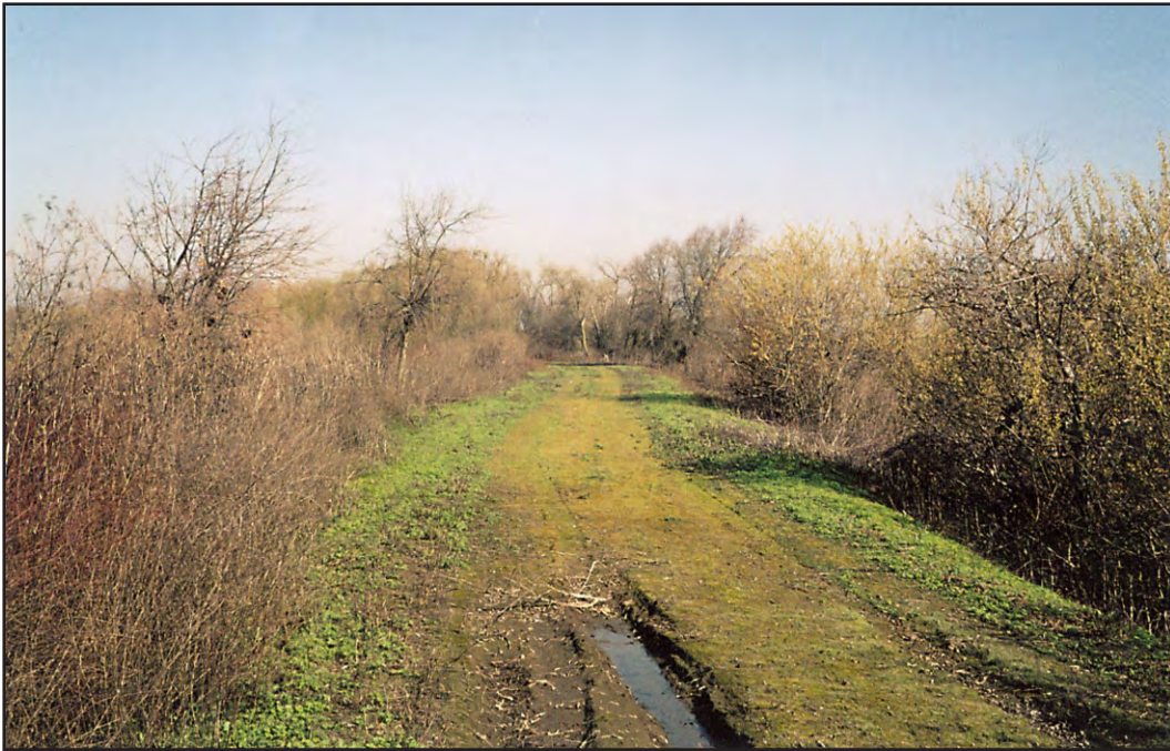
Figure 5-5.9. View of McCormack-Williamson Tract east levee, looking north. This levee would be degraded and armored as a weir under Alternatives 1-A through 1-C.
