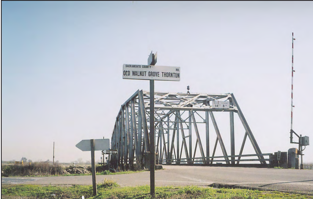
Figure 5.5-4. View of Millers Ferry Bridge, looking southeast at the intersection of Walnut Grove–Thornton Road and Old Walnut Grove–Thornton Road. This bridge would be subject to retrofit or replacement under Alternatives 2-A through 2-C.
