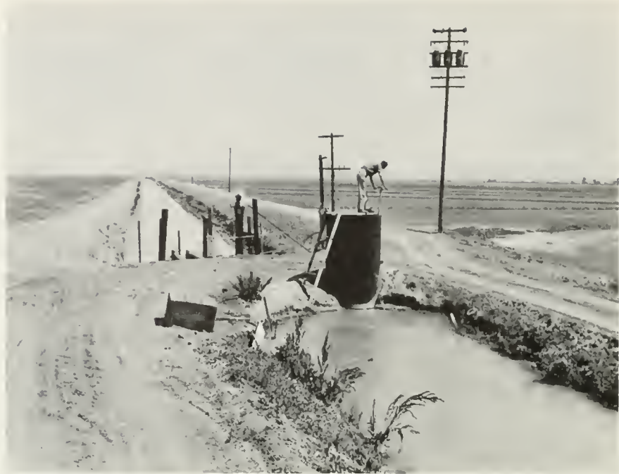
Many of the pumps are located on feeder canals some distance from the main drainage canal.
