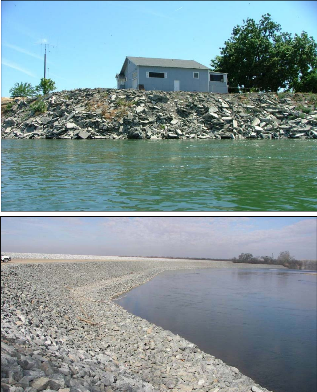
Figure 2. Example of two armored banks on the Sacramento River. The upper photo is private (and likely unpermitted) rubble, installed by landowner to protect property. The bottom photo is an example of almost 0.8 miles of permitted rock installed in 2007 on the riverbank with additional rock placed upslope on the levee. Bank Swallows were active on this previously erodible bank for most of the survey period. Photo credit D. Garcia 2007
