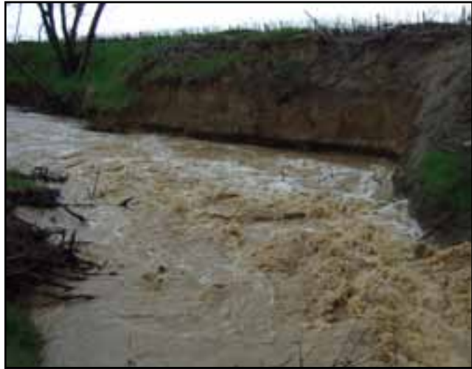
Sedimentation and erosion in a seasonal creek (Photo: Jack Alderson)
