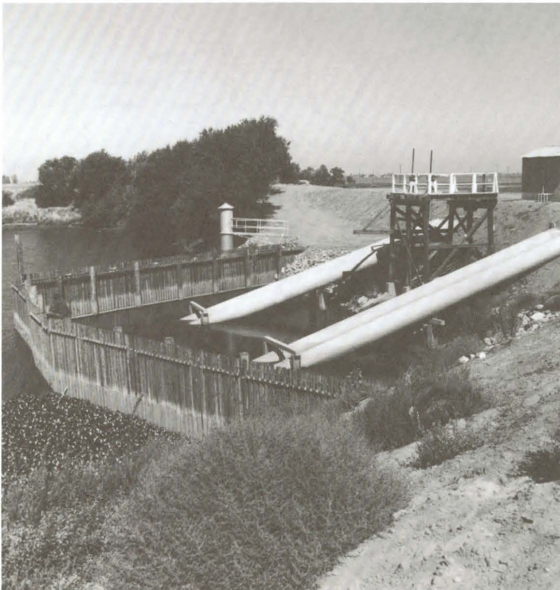
Siphon at Tom Paine Slough, installed as part of a settlement contract to improve water quality in a portion of the South Delta Water Agency.
