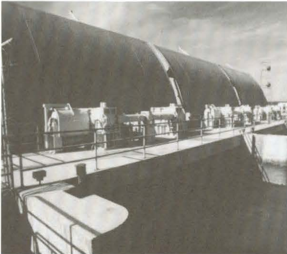
The Suisun Marsh Salinity Control Gates began operating in 1989. Each of the three gates measures 36 feet wide by 28 feet high and operates electronically to improve water quality in the marsh.
