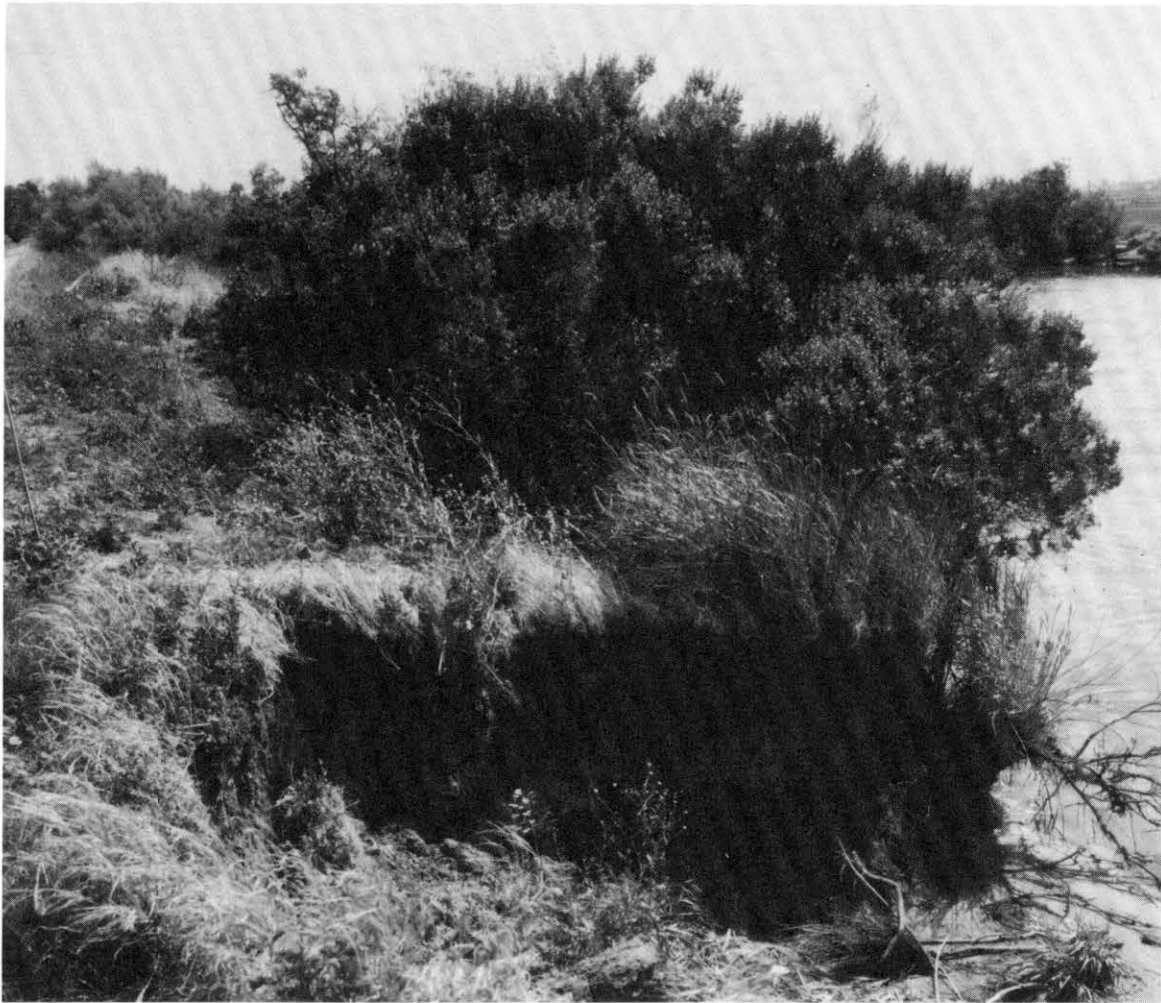
Eroded nonproject levee protecting hundreds of acres of agricultural land and wildlife habitat.
