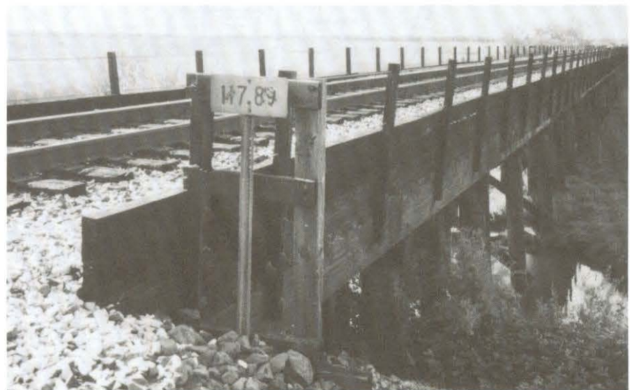
A raised section of the Union Pacific Railroad line northeast of McCormack-Williamson Tract.
