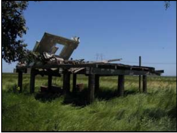
The remains of the Fireman's Clubhouse
