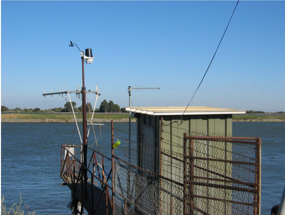
Figure 5.5 - Radar antenna installed at Three-mile slough gage.
