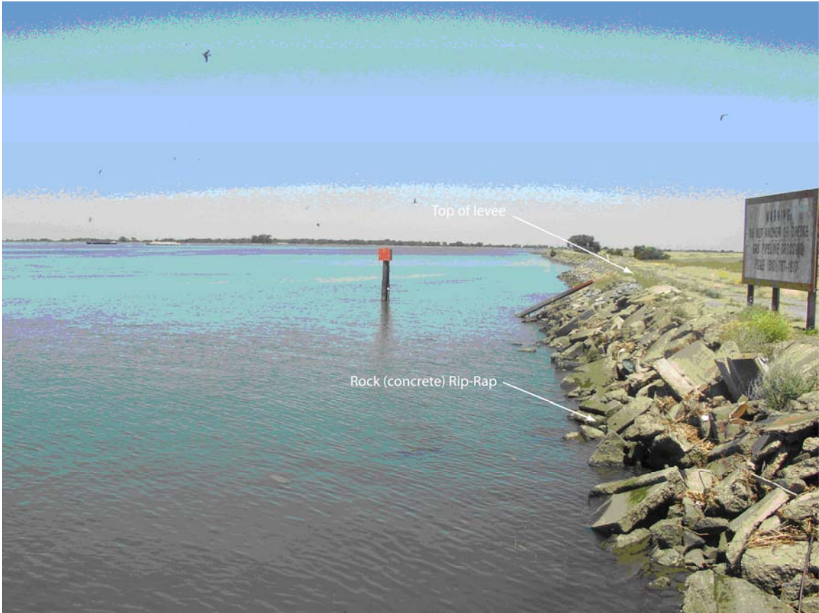
Figure 1.4 – Photograph of Threemile Slough: station TMS. Flow monitoring equipment is mounted on the piling shown.
