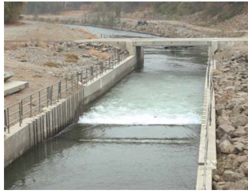
The water control structure resembles a long-throated flume to balance hydraulic conditions
