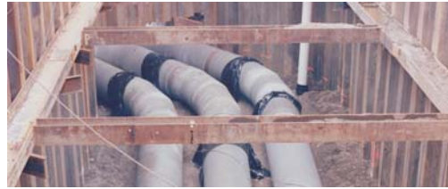
54-inch steel pipe with mortar lined and coated bypass piping to allow tired or stressed fish to bypass structure and be routed downstream of the screens
