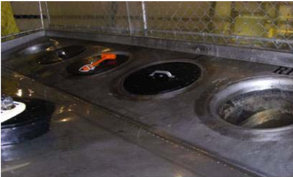
Figure 4-11. Stainless steel tubes that lead to either the holding ponds or the river.
