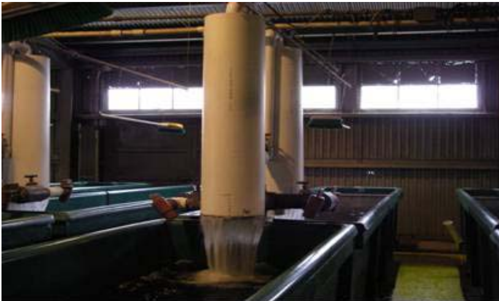
Figure 4-19. Vertical PVC water supply system to NFH Building 1 and 2.
