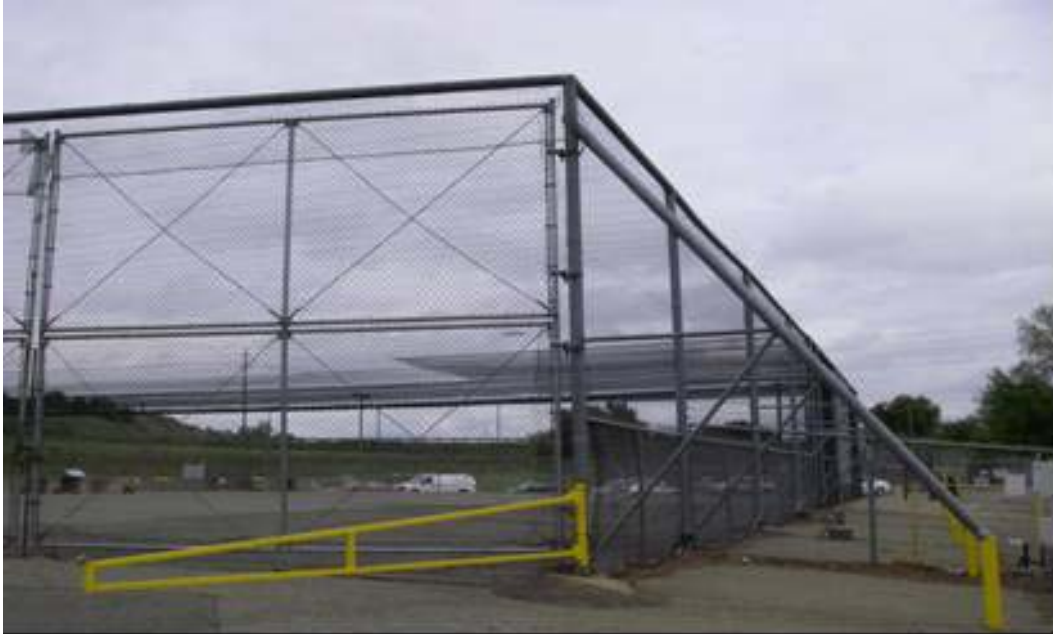
Figure 4-21. Chain link and wire mesh enclosure surrounding the raceways.
