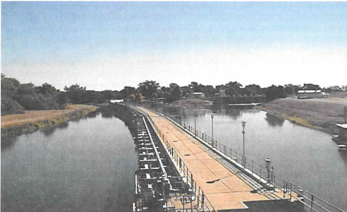
Figure 1. SCADA allows GCID to monitor the activities of its 1,100-foot long fish screen. The pump station is located directly behind the fish screens.
