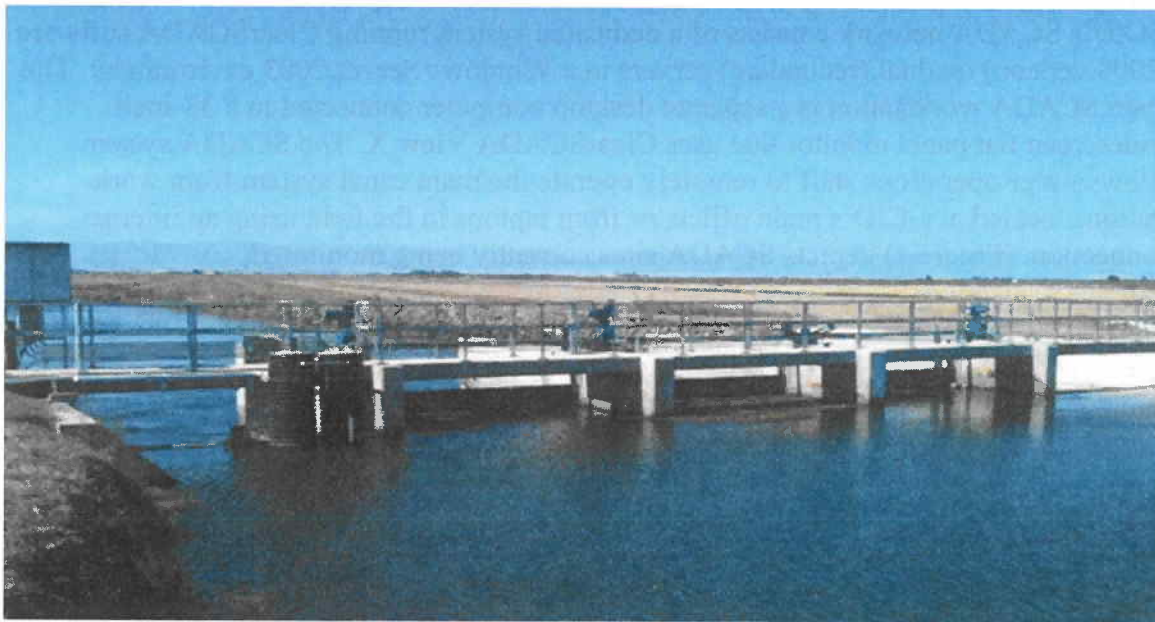
Figure 3. Typical check structure along the main canal; SCADA allows the radial gates to move automatically, maintaining a selected or targeted upstream water elevation.
