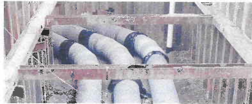
54-inch steel pipe with mortar lined and coated bypass piping to allow tired or stressed fish to bypass structure and be routed downstream of the screens
