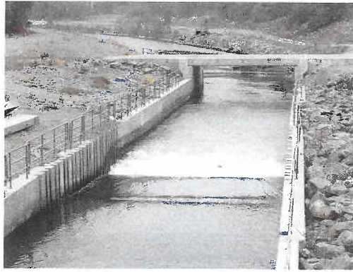
The water control structure resembles a long-throated flume to balance hydraulic conditions
