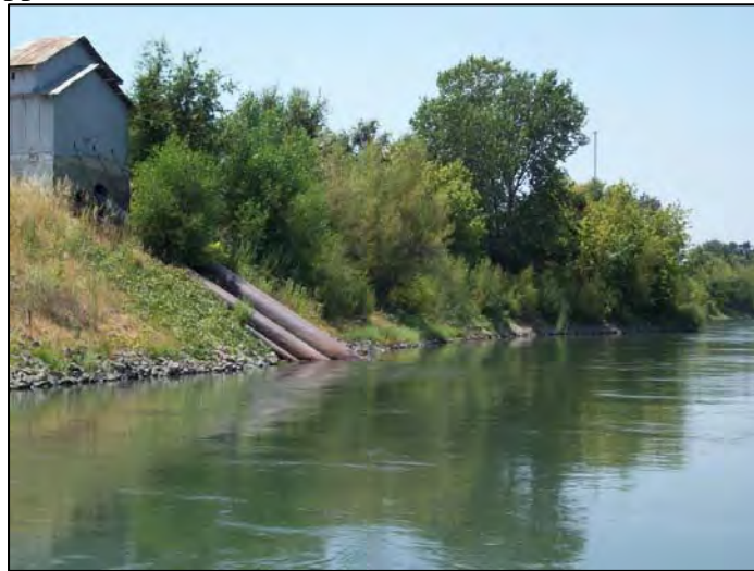
Appendix Figure 51. The Alamo pump intakes looking in an upstream direction.
