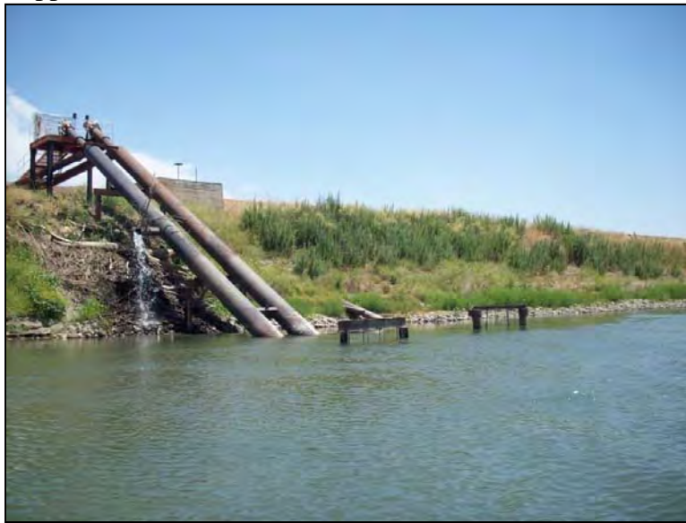
Appendix Figure 30. The Oji pump station intakes looking in a downstream direction.
