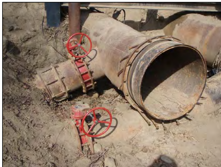
Figure 119. Flow bypass valves (red) at the Sycamore diversion. The two large-diameter pipes on the right lead to the Sycamore canal through a levee. Each pipe has a separate flow bypass valve on the left that can be used to route excess pumped flow back to the Sacramento River. The left intake pipe is disconnected for pump maintenance.
