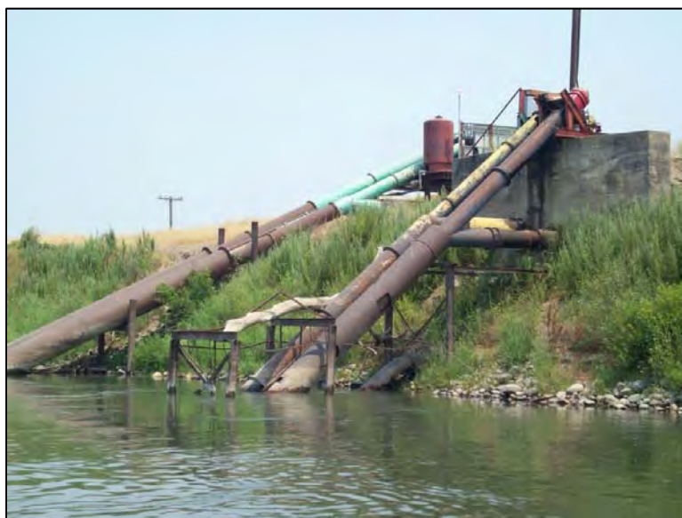
Appendix Figure 72. The Cranmore pump intakes (foreground) looking in an upstream direction.
