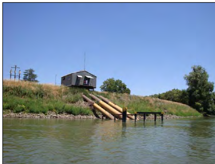
Appendix Figure 44. The Portuguese Bend pump station intakes looking in a downstream direction.
