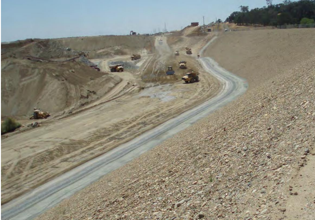
Figure G14. Two-stage filter being installed within overlay at MIAD in California. The filter is the light gray band crossing the picture from the lower left corner.
