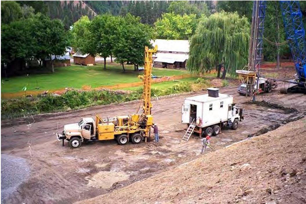
Figure G2. Verification testing with SPT and CPT to confirm sufficient densification by Stone Column Construction at Salmon Lake Dam. Stone column equipment appears at the far right side of the photograph.
