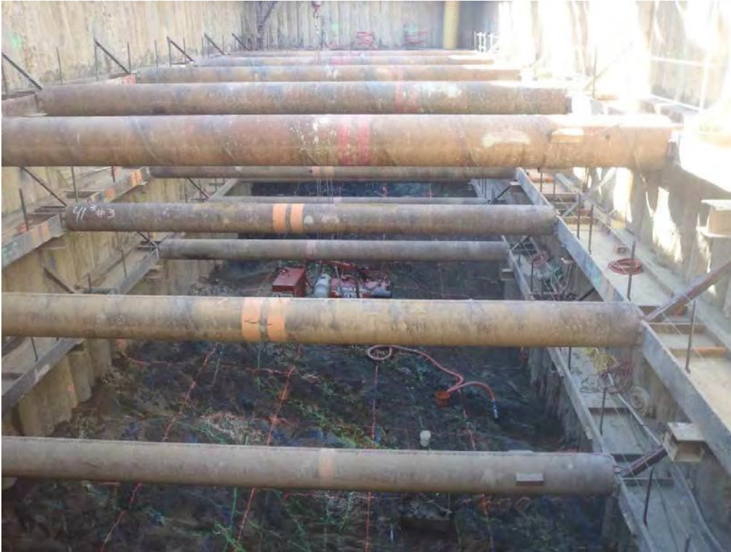
Figure G4b. Excavation bracing for the key block at MIAD, Folsom, California (2011).
