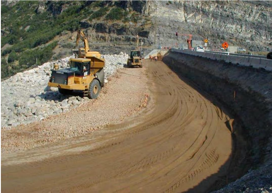
Figure G18. Placement of flowthrough rockfill, transition, and filter zones, downstream to upstream (left to right), Pineview Dam modification, Utah.
