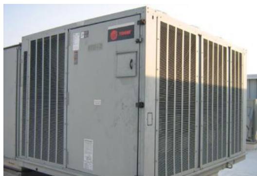
Rooftop HVAC system
