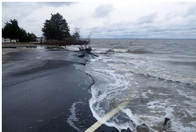
Flood damage from Hurricane Sandy at Assateague Island National Seashore Park (Virginia)
