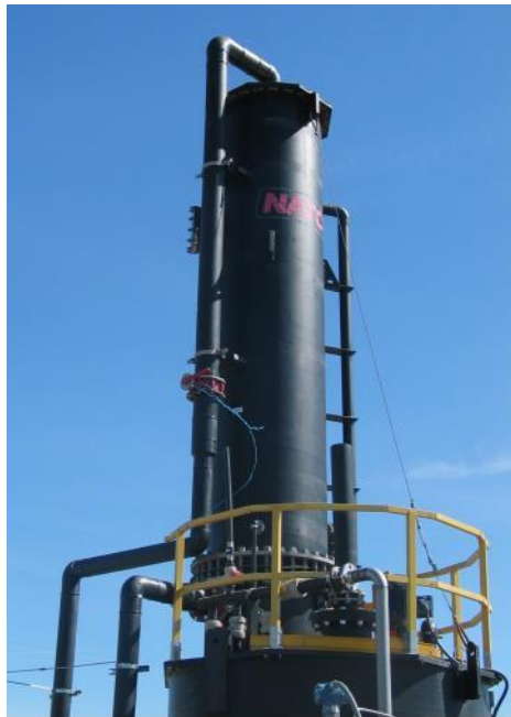
Dairy gas cleanup system (gas scrubber)
