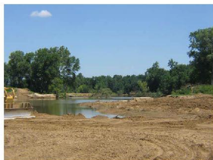
Fig. 3 Crater lake extending through 100-m levee breach.
