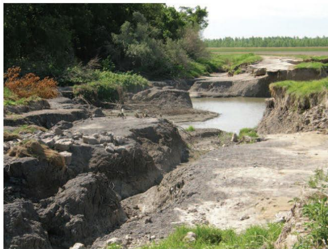
Figure 4 May of 2011 trees falling into channel and undercutting County Road 310.
