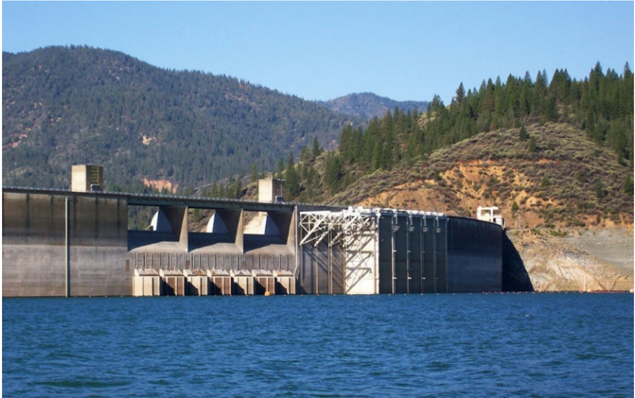
Shasta Dam Temperature Control Device
