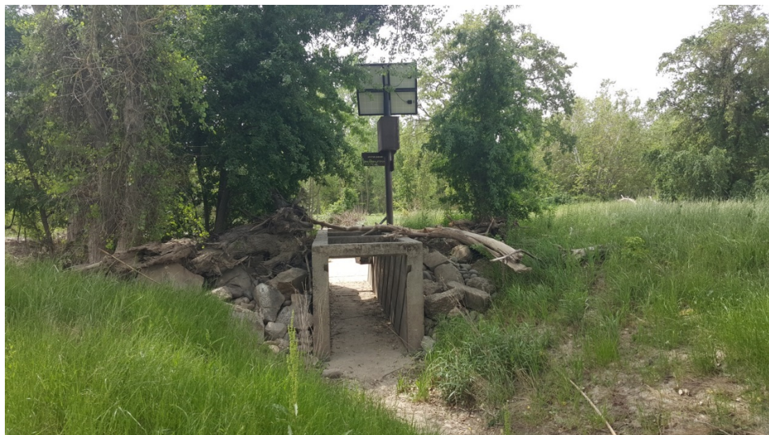
Figure 14-6. Fremont Weir fish ladder intake channel – photo taken from the river side looking south at the intersection of the fish ladder with the existing intake channel (May 2016).
