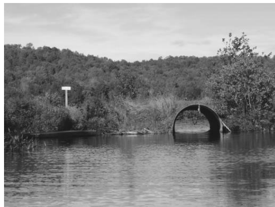
Figure 9.5. Culvert installed on an embankment built across the back of a cove. Photo credit: www.slideshare.com .
