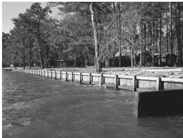
Figure 5.19. Bulkhead designed to control wind-induced shore erosion. Photo credit: M&M Marine Construction, Queenstown, Maryland.
