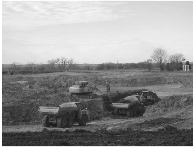
Figure 3.10. Excavation of accumulated sediment at a Nebraska reservoir. Photo credit: M. Porath, Nebraska Game and Parks Commission, Lincoln.
