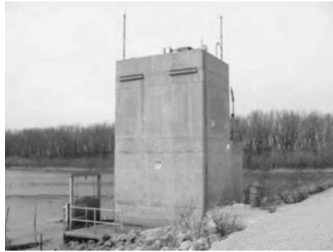
Figure 9.7. Permanent pumping station at the Andalusia Refuge, Pool 16, Upper Mississippi River. Photo credit: USACE, Rock Island District.
