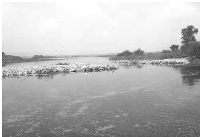
Figure 9.4. Partial closure structure at the Weaver Bottoms secondary channel, Pool 5, Upper Mississippi River. Photo credit: USACE, Rock Island District.
