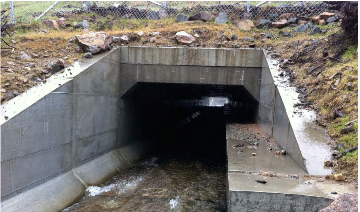
Figure 79: A cast-in-place concrete stream passage with a mammal shelf, that could be enhanced for use by herpetofauna with addition of directional fencing. Image: Tony Clevenger
