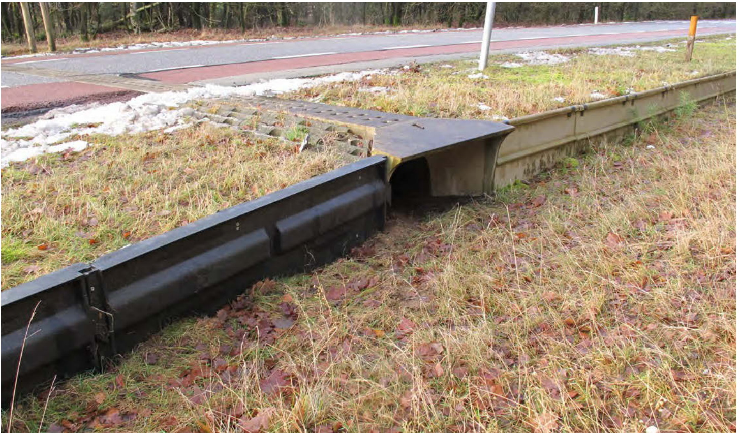
Figure 48: Guide walls for small snakes and lizard species on a single lane road with cycle path. Attached to a Type 5 (20 in/0.5 m wide) micro-passage, is a molded plastic barrier on the left hand side and a polymer concrete barrier on the right hand side. Both barrier types are circa 20 in/0.5 m above ground. Image: Tom Langton
