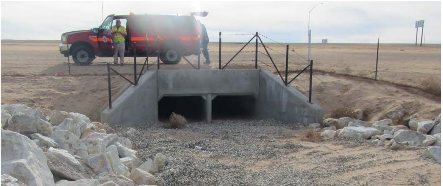
Figure 28: A new culvert built under State Route 58 in southern California (Hinkley Highway Re-alignment Project, Caltrans District 8). Adjustments will be needed to join wire fencing to the entrance of the passages and to make the rip-rap safe, so desert tortoises do not get trapped in it.
