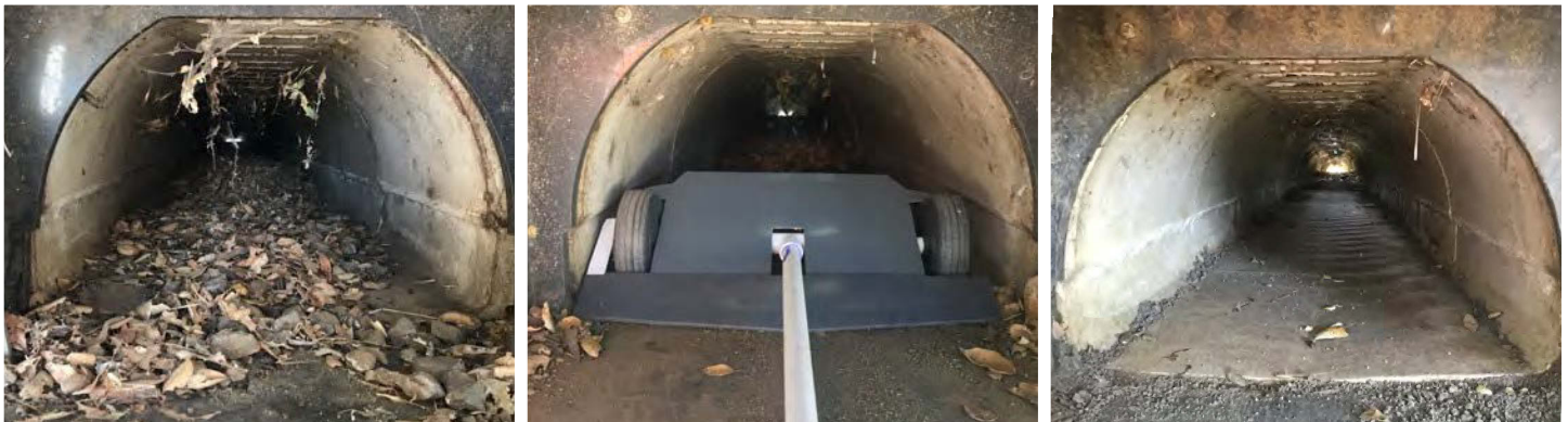
Figure 71: Blown leaves may in some locations fill and become compacted in a small passage thus reducing wildlife use. An extending pole device can clear them as shown in this slotted surface passage.
