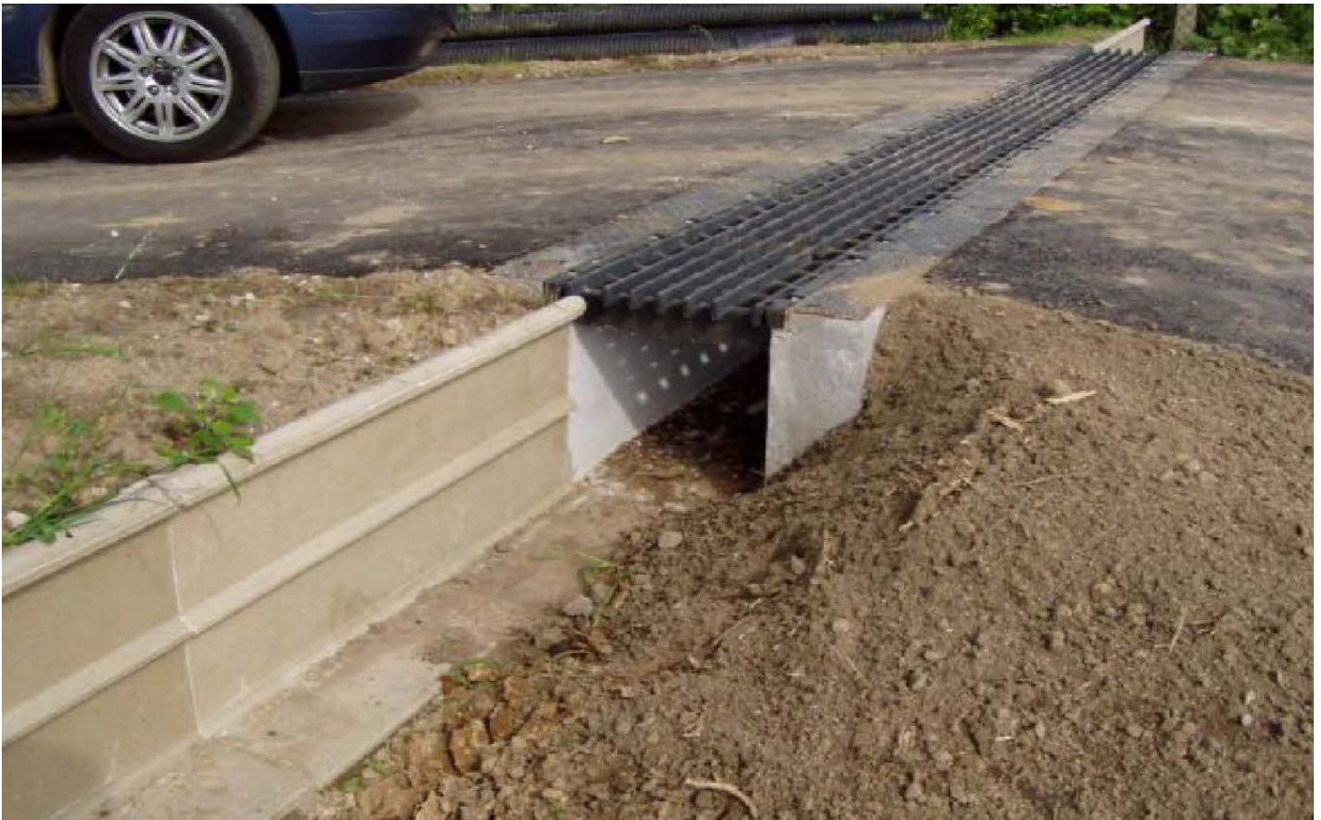
Figure 60: A purpose-made 'stop grid', built where a side road approaches a main road in a herp migration location. Gratings may be made with wider gaps but must conform to road regulations. Image: ACO
