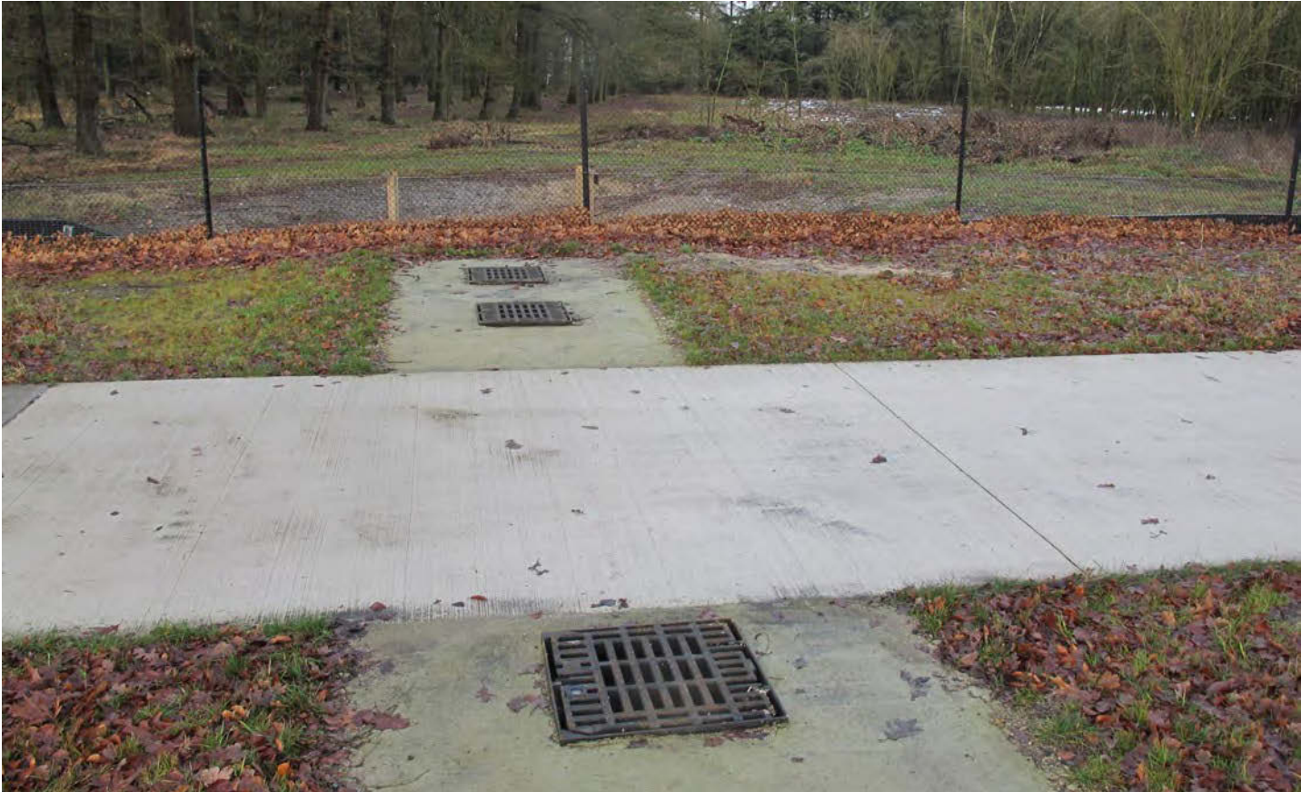
Figure 31: Located on the far side of the road shown in Figure 30 and either side of the cycle lane is a series of cast steel gratings placed within the roof of the wildlife passage to allow entry of light and moisture. Image: Tom Langton
