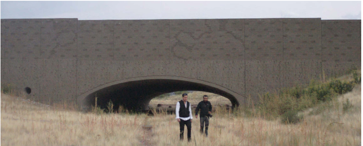
Figure 24: A Type 2 underpass in the Sonoran Desert in Arizona, constructed for passage by deer and bighorn sheep. The passage crosses under a 6-lane road with a median. It is a purpose-built, 50 ft wide, 12 ft high, and 190 ft long (15.2 m wide, 3.6 m high and 58 m long) structure is located at Oracle Road, near Tucson, Arizona. Image: Tony Clevenger.
