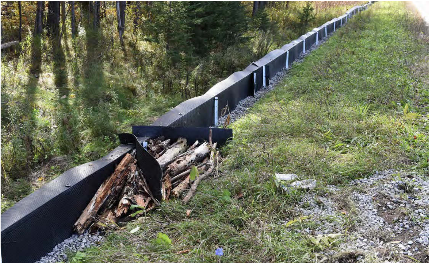
Figure 62: A jump-out constructed within a section of solid HDPE sheet fence, constructed along a road edge. The jump-out is outfitted with decaying logs to form a ramp for small turtle species and it directs them to the safe side of the barrier. Image: Animex fencing
