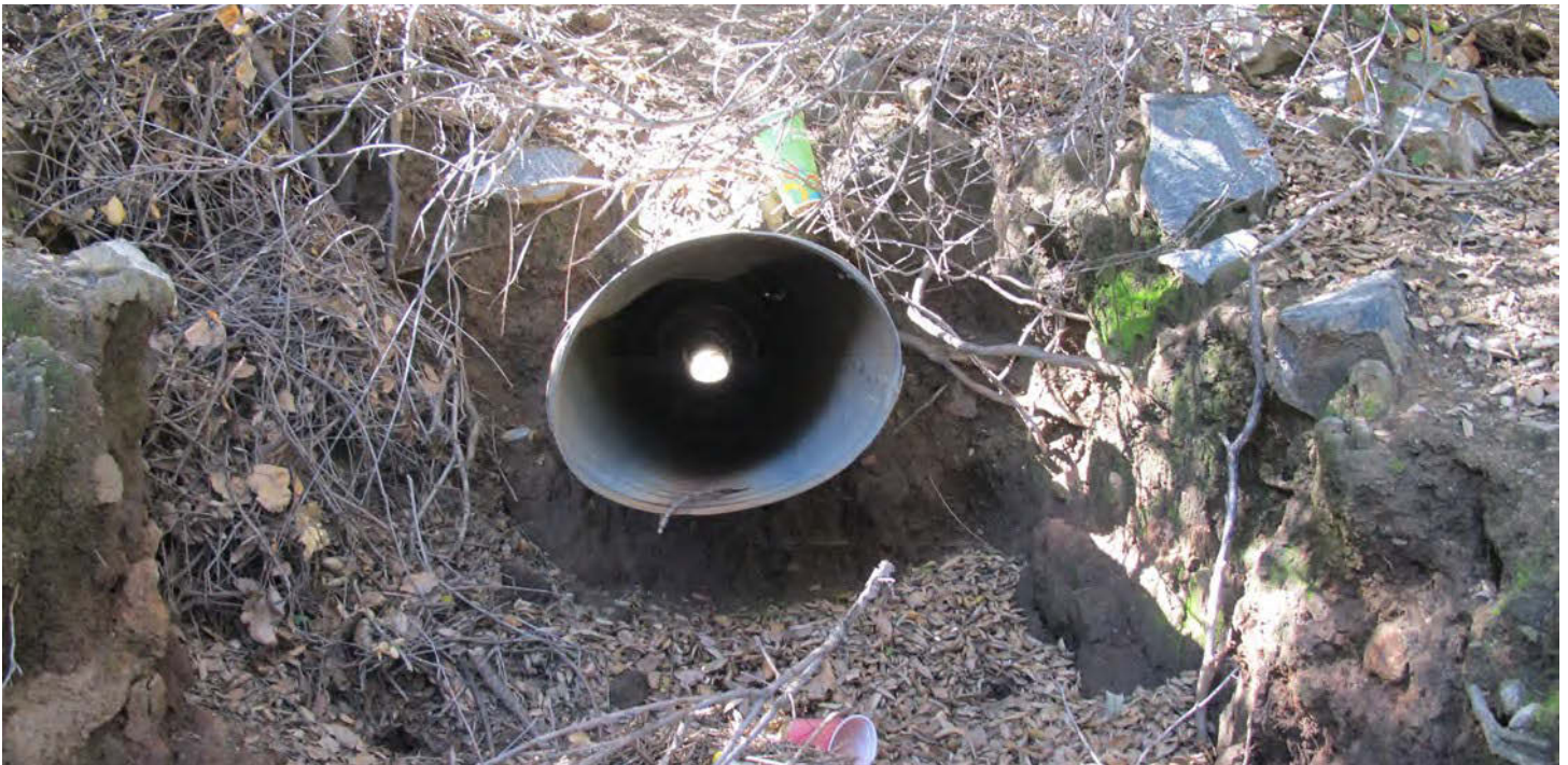
Figure 38: There are many small cross-road steel drainage culverts on California roads, such as this elliptical shaped steel culvert near San Diego. This culvert was built during the last century and is nearing time for refurbishment. This type of scenario offers an opportunity for culverts to be adapted for safe wildlife passage as well as for road drainage purposes. See also Chapter 9. Image: Tom Langton
