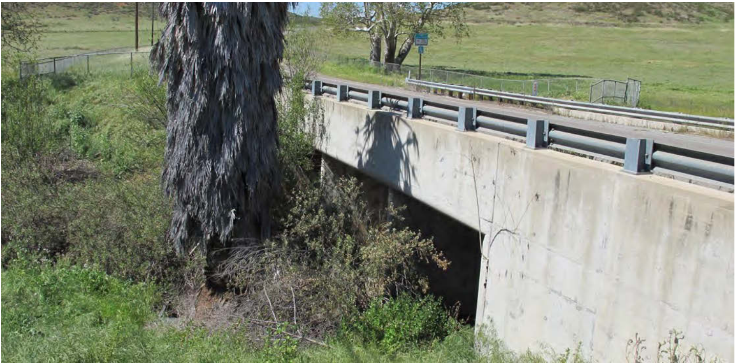
Figure 26: Image shows a 30 ft/9.1 m Type 3 concrete temporary stream bridge along Campo Road/Highway 94, San Diego County, south of San Diego. The bridge has three 10 ft × 10 ft concrete chambers and was built without specific wildlife goals. Image: Tom Langton
