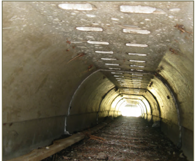
Photo 8. ACO open-top tunnel allowing light into tunnel. © Kari Gunson
