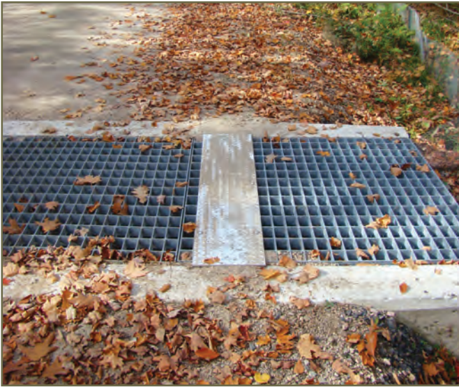
Photo 3. Open-grate tunnel at Killbear Provincial Park, Ontario. © K. Gunson
