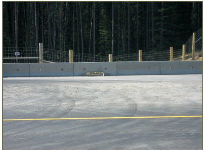
Photo 61. Jersey barrier with gaps at the road surface ©K. Gunson
