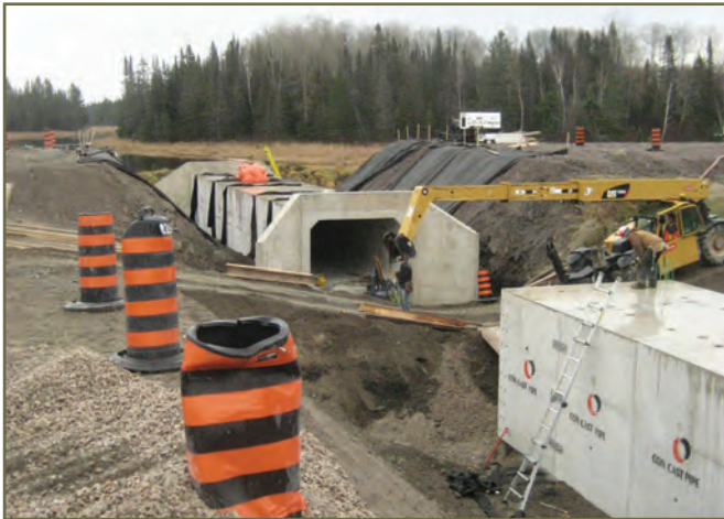
Photo 20. 3.4 x 2.4 m concrete box culvert connecting wetland habitat used by turtles on highway 69. © K. Gunson
