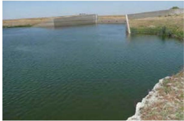
The drop structure on the Mariposa Bypass helps control the channel grade near its downstream end
