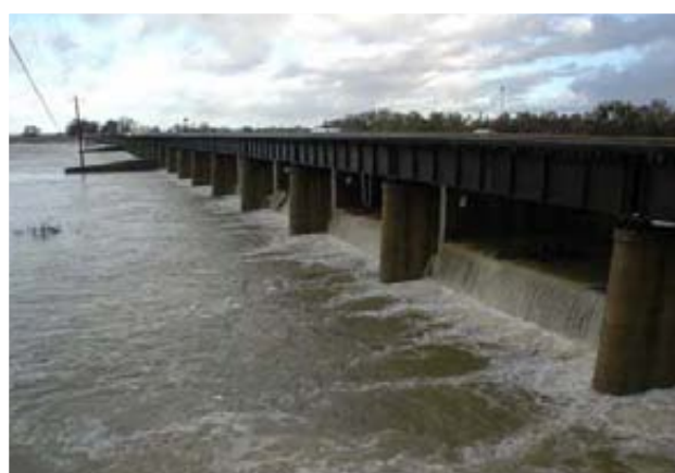
The Sacramento Weir is the only weir that requires manual operation for flow release
