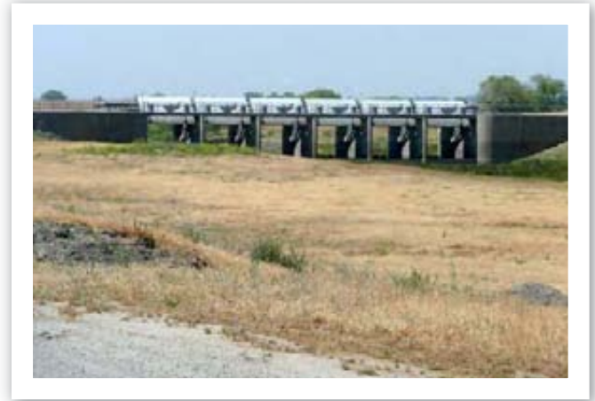
SPFC facilities in the San Joaquin River Basin include the Eastside Bypass Control Structure
