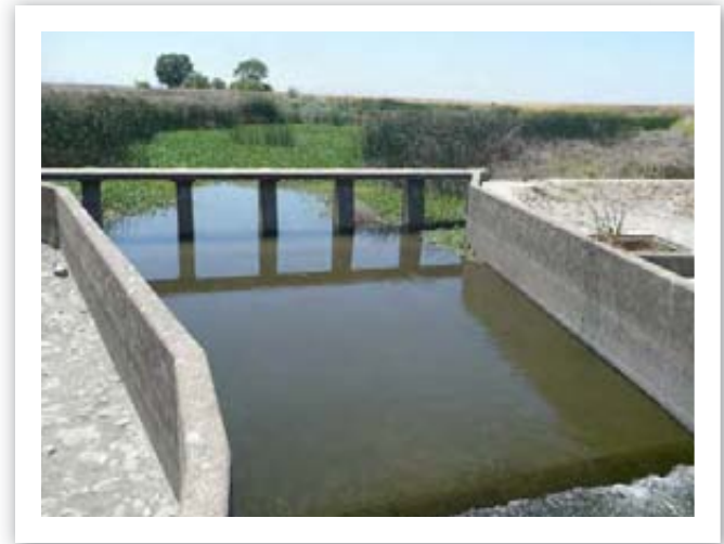
The Sand Slough Control Structure spills San Joaquin River water into the Eastside Bypass
