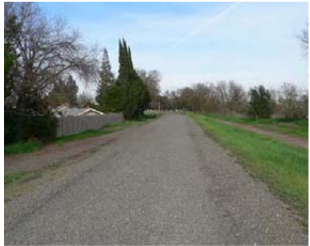
The American River right-bank levee extends from high ground near Carmichael Bluffs
