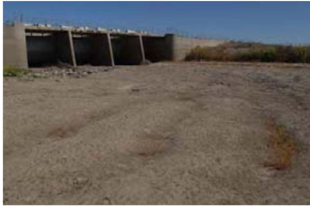
Levees line the channel downstream from the Chowchilla Canal Bypass Control Structure
