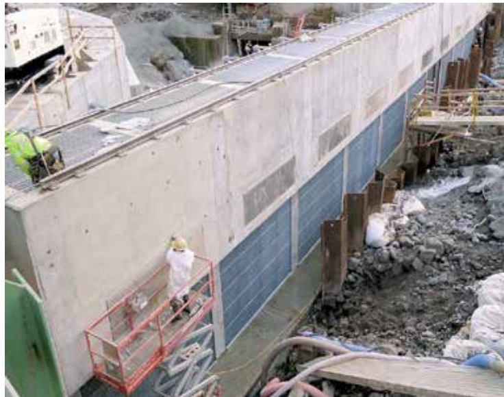
2552 2553 Figure 6-3. Picket barrier panels under construction at the Slide Creek tailrace barrier located on 2554 the North Umpqua River, Oregon
