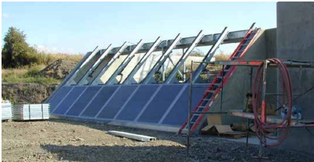
4608 4609 Figure 10-2. Bankline screens at the Garden City-Lowden 2 diversion on the Walla Walla River 4610 near Touchet, Washington, under construction
