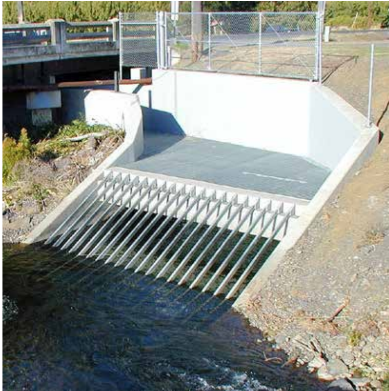
2103 2104 Figure 5-12. Sloping coarse trash rack on a fishway exit channel
