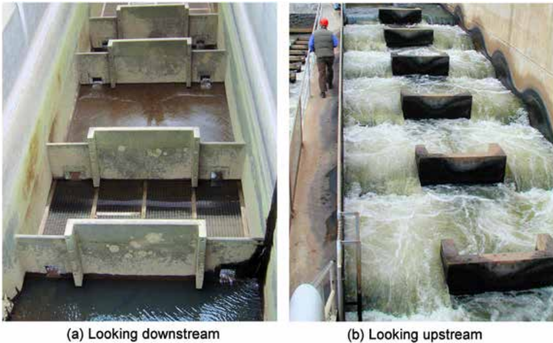
1785 1786 Figure 5-9. Overhead views of Ice Harbor-style weir and orifice fish ladders
