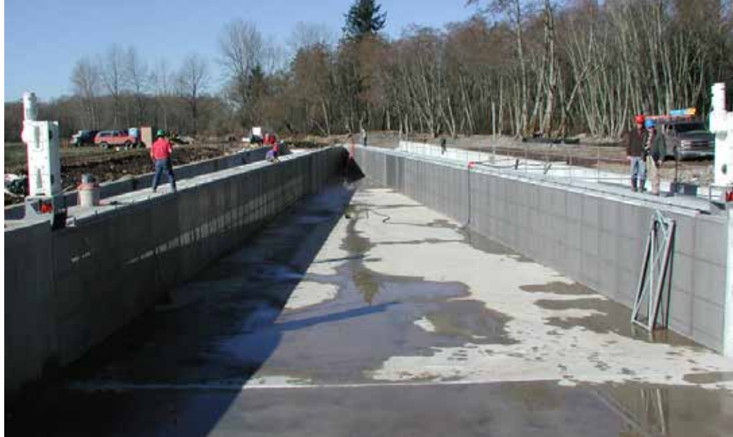
4629 4630 Figure 10-5. Vertical plate screen facility under construction in a diversion canal located on the 4631 Santiam River near Stayton, Oregon
