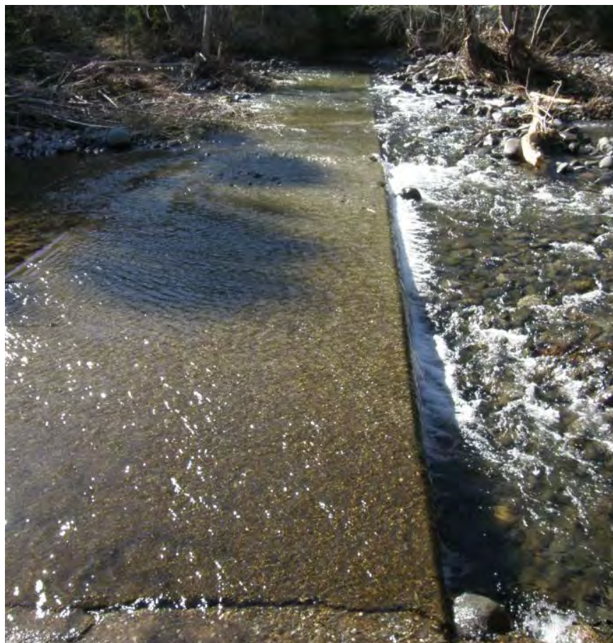
Figure 19 Antelope Creek lower slab post 2014 high flows
