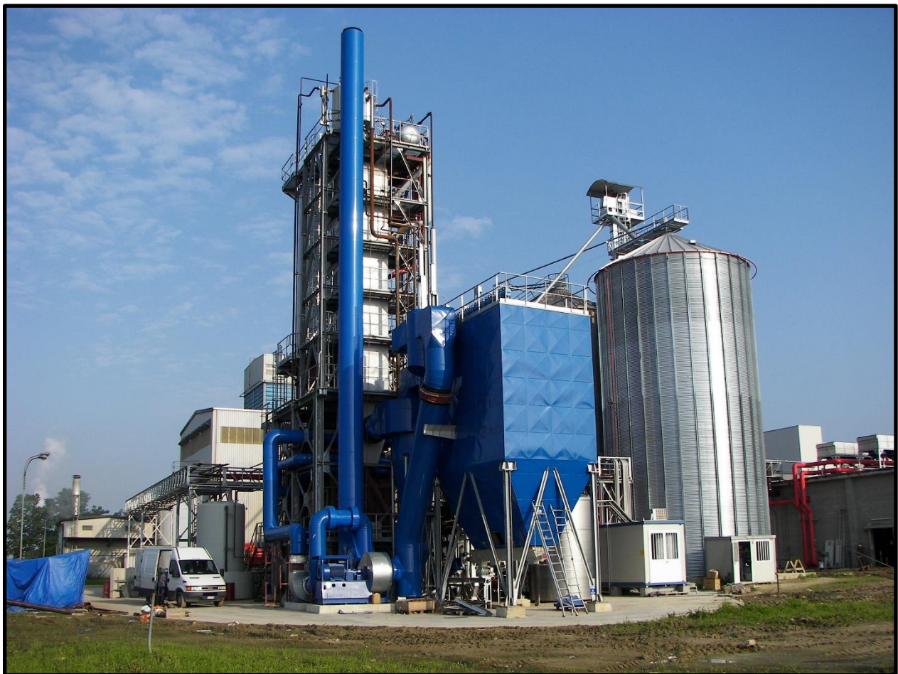
Figure 2 - Reference Rice Hull Powerplant Facility in Northern Italy
