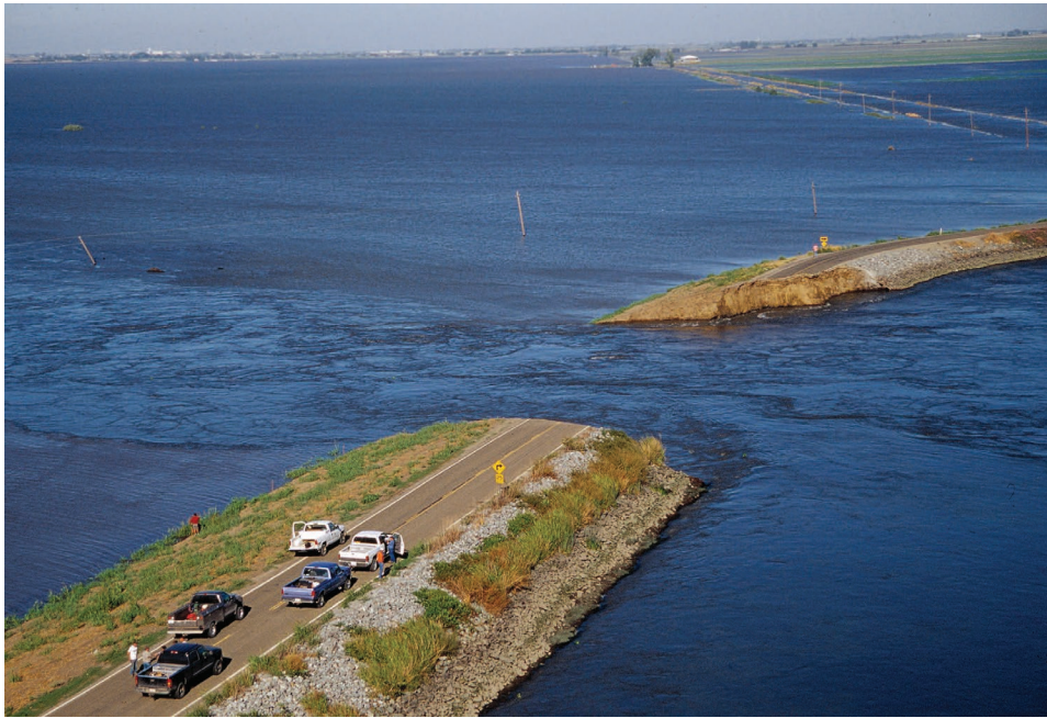
Figure 6-1 Photo of Jones Tract Levee Failure (June 4, 2004)
