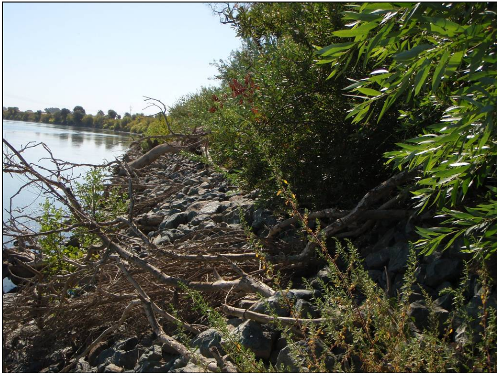
Site 85.6R, Photo-point 1. Repair site with a no bench design. Photo taken September 2009.
