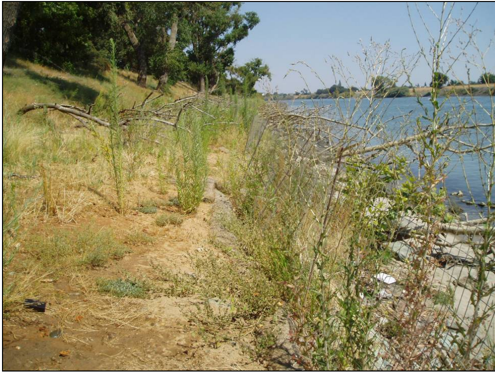
Site 43.7R, Photo-point 4. Repair site with 10:1 slope design. Note that a large portion of the installed instream woody material is above the water level. Photo taken August 2008.
