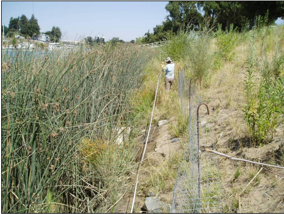
Site 26.9L, Photo-point 1. Repair site with Dietl ditch design. Standing on the bank side of the ditch, facing north. Note the large abundance of aquatic vegetation within the Dietl ditch. Photo taken August 2008.
