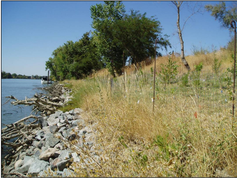
Site 50.2L, Photo-point 1. Repair site with a no bench design. Photo taken August 2008.
