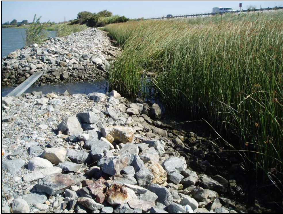
Site 10.7L, Photo-point 4. Repair site with Dietl ditch design. Note the large abundance of aquatic vegetation within the Dietl ditch. Photo taken September 2008.
