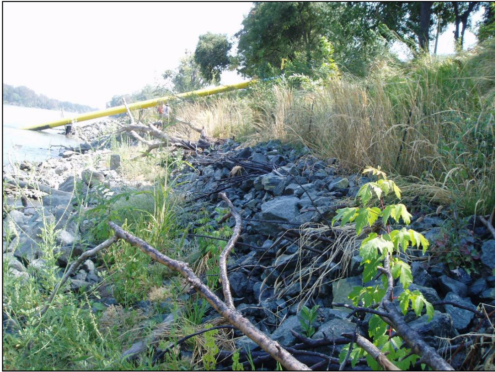
Site 69.9R, Photo-point 1. Repair site with a no bench design. Photo taken August 2008.
