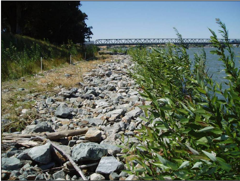
Site 12.7L, Photo-point 2. Repair site with bench design. Note the early development of overhanging shade from the willow plantings adjacent to the channel. Photo taken August 2008.
