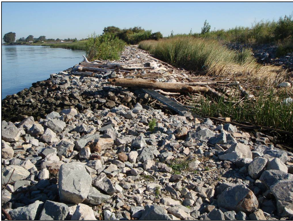
Site 10.7L, Photo-point 4. Repair site with Dietl ditch design. Note the large abundance of aquatic vegetation within the Dietl ditch. Photo taken October 2009.
