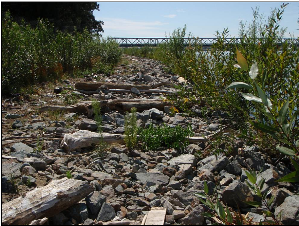
Site 12.7L, Photo-point 2. Repair site with bench design. Note the continued development of overhanging shade from the willow plantings adjacent to the channel. Photo taken September 2009.
