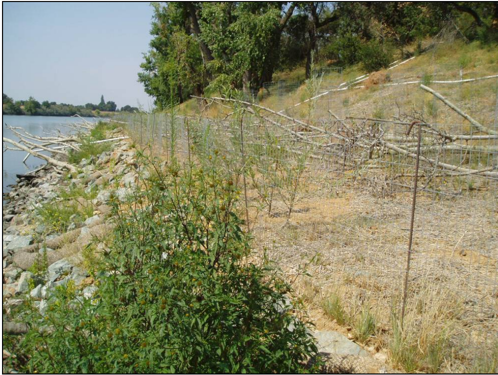
Site 44.7R, Photo-point 4. Repair site with 10:1 slope design. Note that a large portion of the installed instream woody material is above the water level. Photo taken August 2008.
