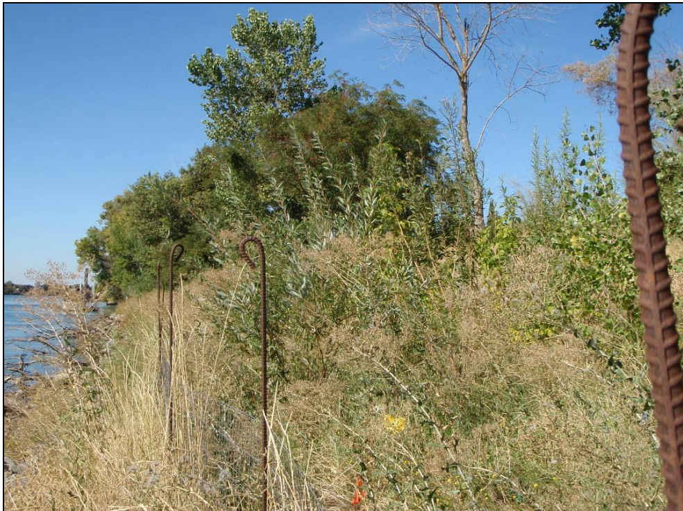
Site 50.2L, Photo-point 1. Repair site with a no bench design. Photo taken October 2009.
