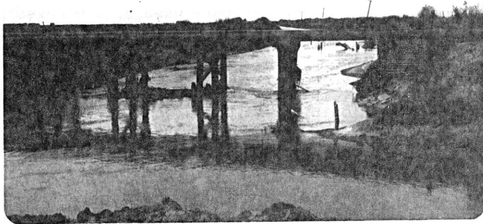
HARBISON ROAD BRIDGE DEBRIS
