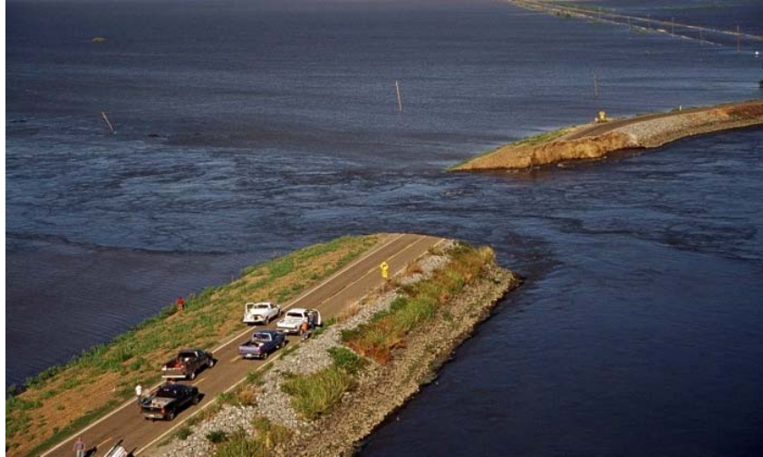
Levee break on Upper Jones Track, June 3, 2004. Photo: California Department of Water Resources.
