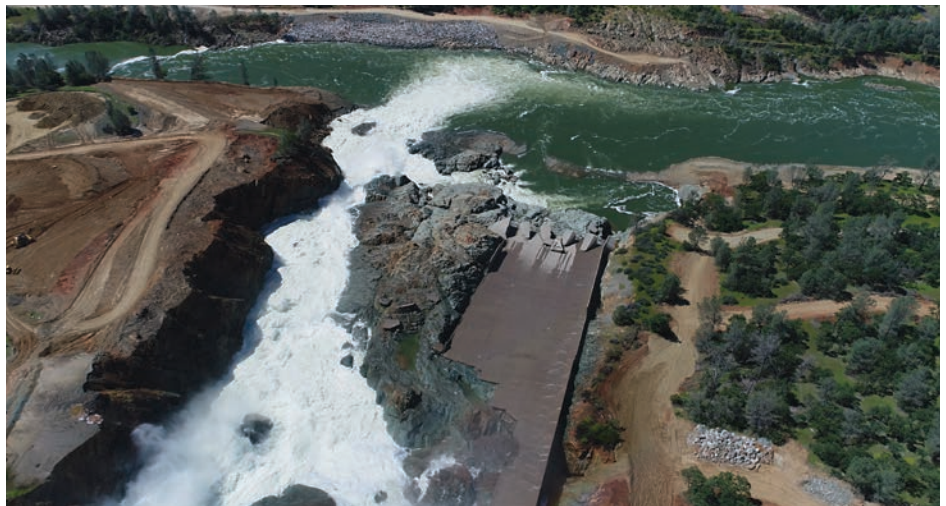
The Oroville spillway failure.
